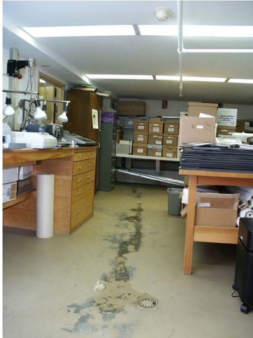
Figure 6: Regular drainage problems in the workshop.
