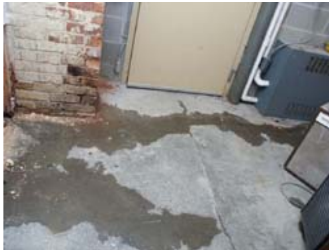
Figure 7: Regular drainage problems in the electrical room (next to the Vault).
