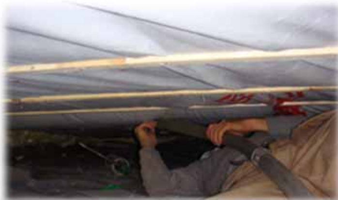
A weatherization technician installs blown in insulation into the floor system pictured above.
