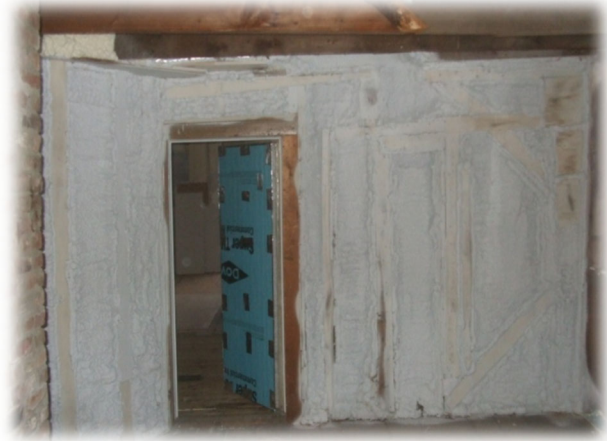
Above, spray foam was utilized to separate an unheated storage area from the rest of the home.
