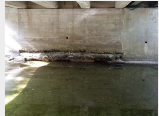
Location of Abutment Undermining
