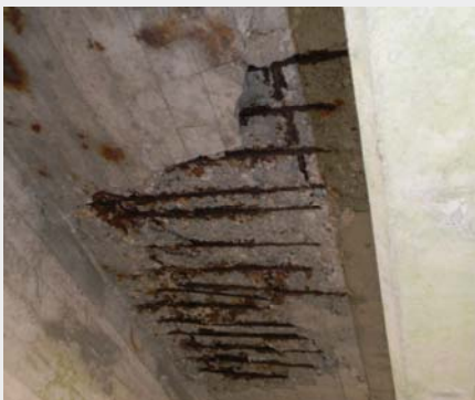
Spalling and Exposed Rebar
