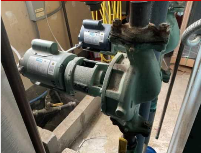
13 - HOT WATER DISTRIBUTION PUMPS
