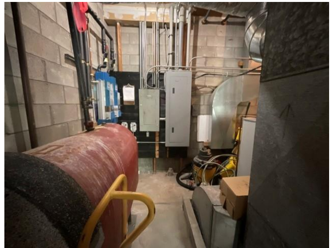
16 - MAIN ELECTRIC ROOM
