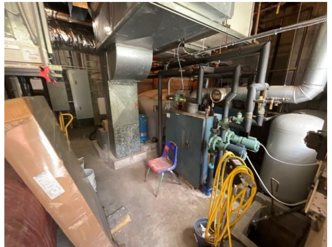
10 - MAIN MECHANICAL ROOM
