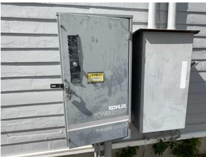
17 - TRANSFER SWITCH FROM GENERATOR
