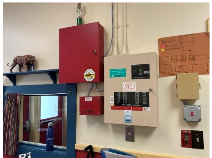
18 - FIRE ALARM SYSTEM OFFICE
