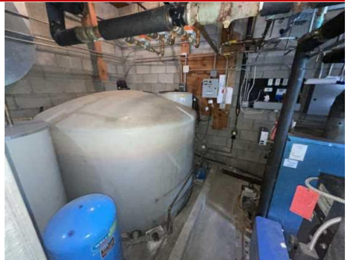
14 - WATER STORAGE TANK FROM WELL
