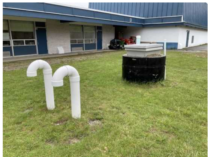
18 - UNDERGROUND WATER TANK
