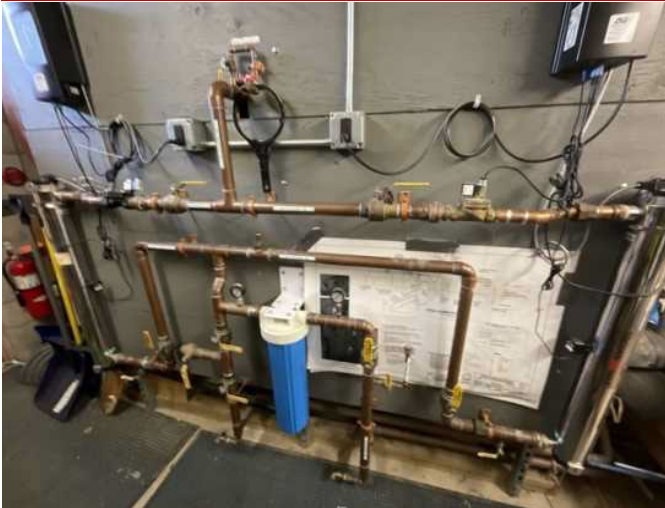
19 - CHLORINE FREE WATER SANITATION SYSTEM
