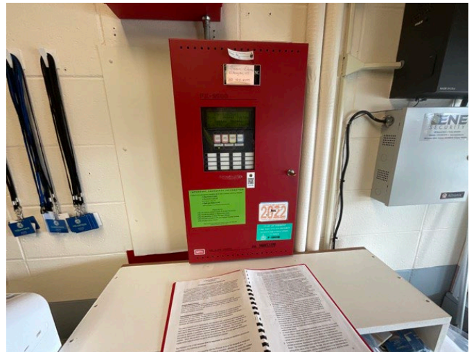
22 - FIRE ALARM ENUNCIATOR PANEL
