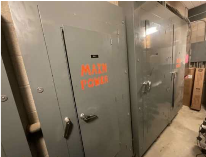
21 - MAIN ELECTRIC ROOM
