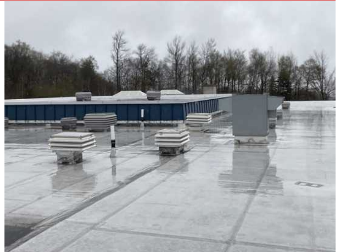
20 - ROOFTOP EXHAUST EQUIPMENT
