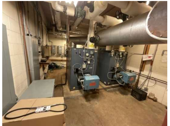
16 - MAIN MECHANICAL EQUIPMENT ROOM
