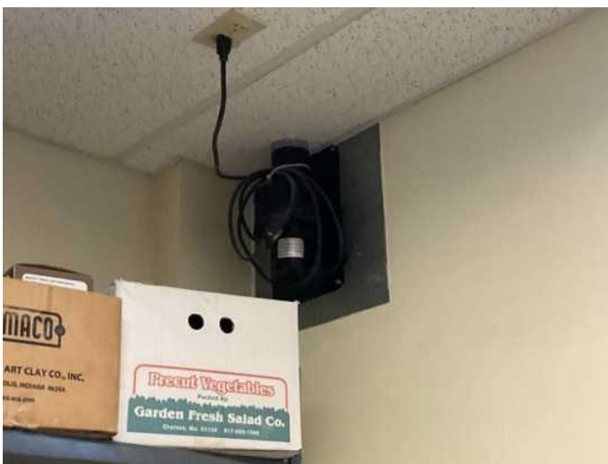
29 - NEW HVAC ASSET
