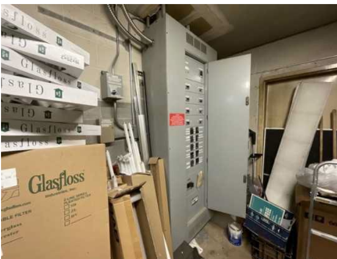
29 - BUILDING MAIN ELECTRICAL SWITCHGEAR
