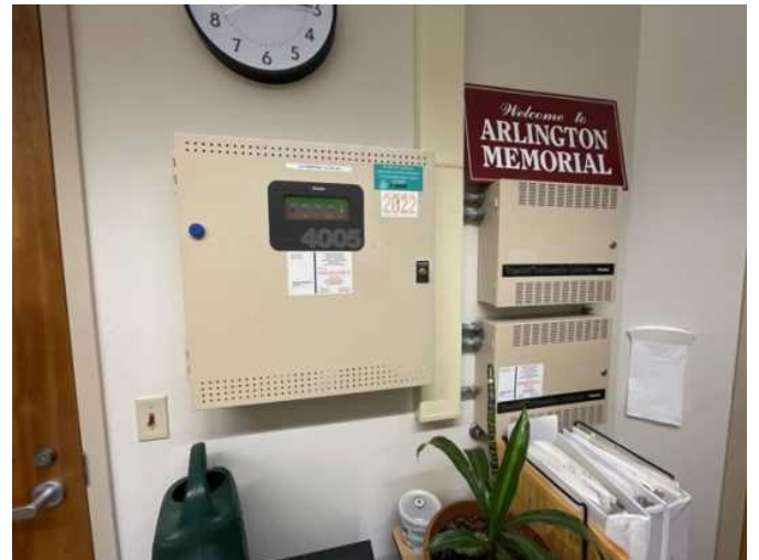
34 - FIRE ALARM PANEL EQUIPMENT
