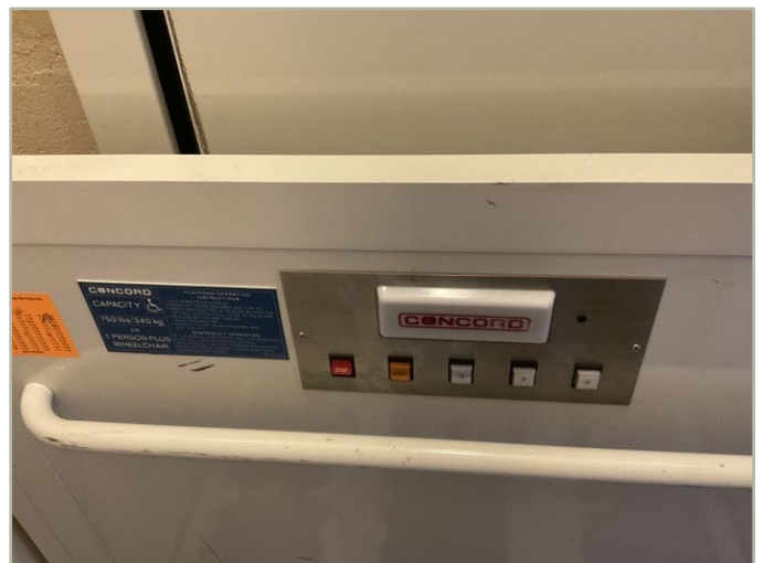
12 - IN-CAB CONTROLS/EMERGENCY CALL PANEL
