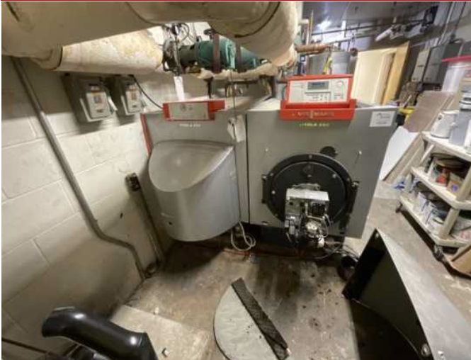
25 - BUILDING OIL FUEL BOILER
