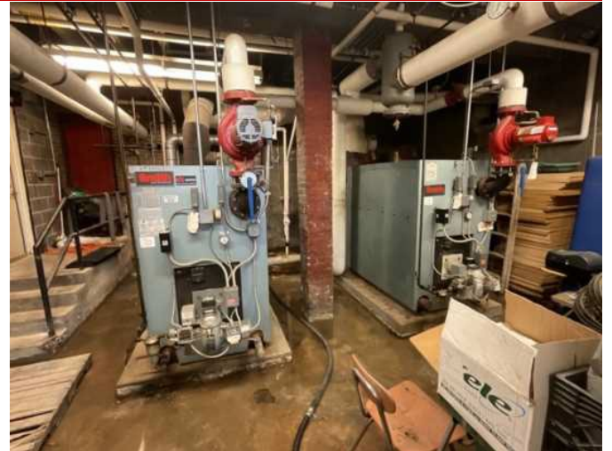
26 - BUILDING OIL FUEL BOILER
