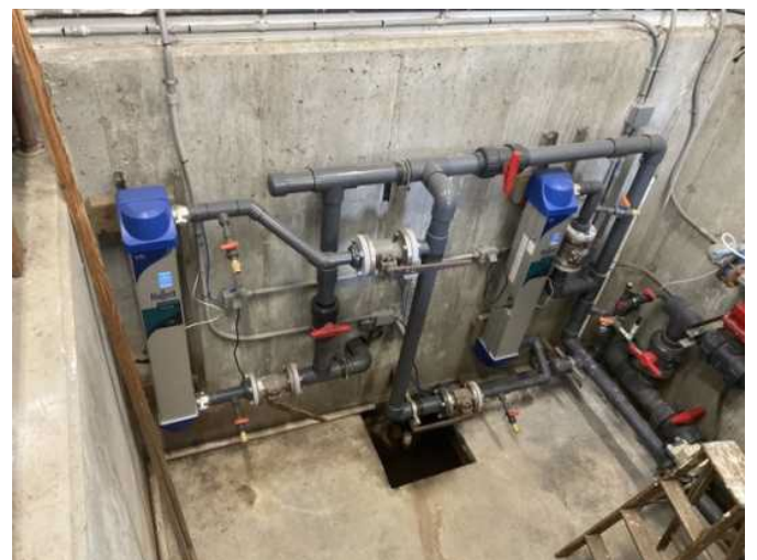
24 - WATER TREATMENT FILTRATION EQUIPMENT
