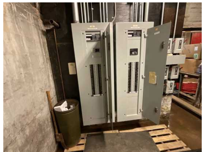
30 - BUILDING MAIN ELECTRICAL DISTRIBUTION P
