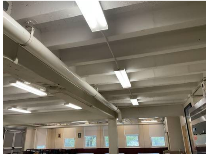
32 - INTERIOR CEILING MOUNTED LIGHTING
