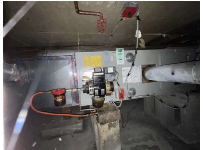
28 - RED BUILDING OIL FUEL FURNACE
