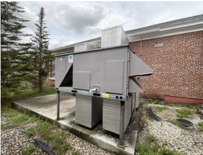
27 - EXTERIOR LOCATED HVAC SYSTEM
