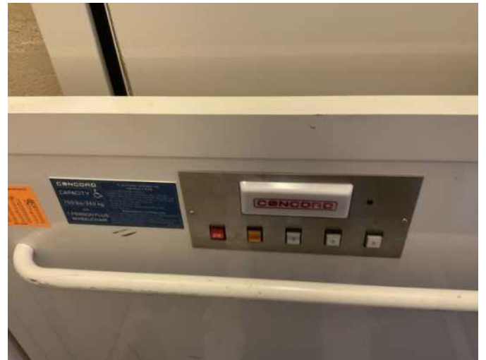
22 - WHEELCHAIR LIFT CONTROL PANEL
