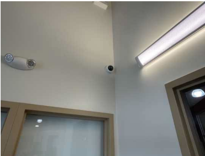
33 - SECURITY SURVEILLANCE CAMERA SYSTEM
