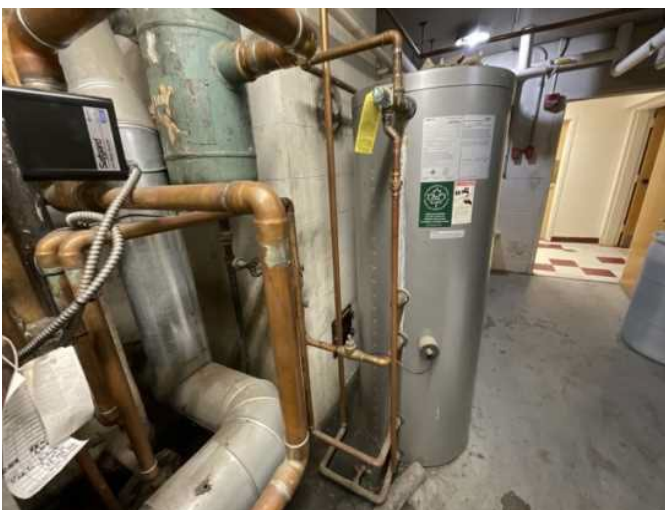
23 - HOT WATER HEATER EQUIPMENT
