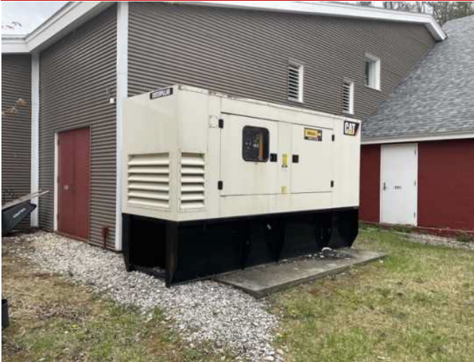
31 - BACKUP DIESEL GENERATOR EQUIPMENT
