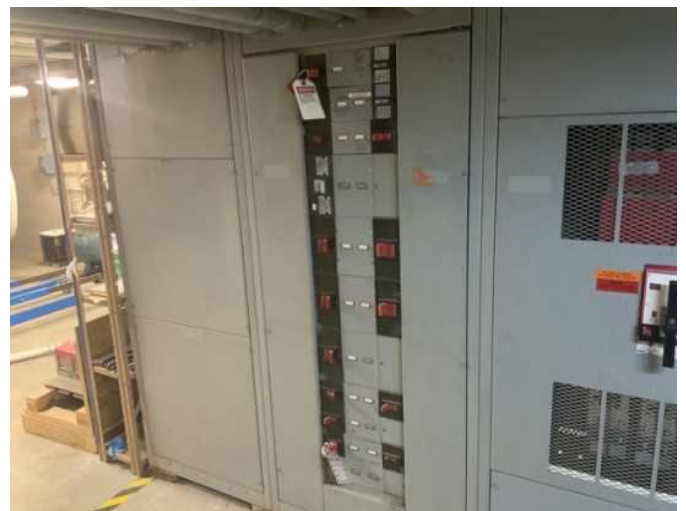
22 - MAIN ELECTRICAL DISTRIBUTION PANEL
