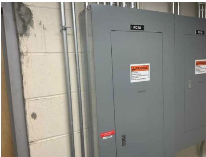
21 - ELECTRICAL DISTRIBUTION PANEL
