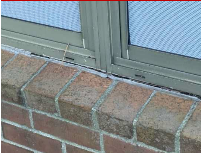
7 - WINDOW CAULKING PULL AWAY
