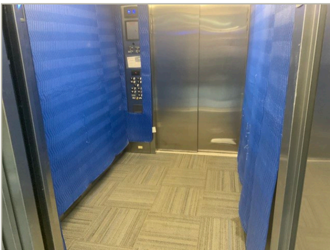
11 - LOBBY VIEW OF CABS, WITH DOORS OPEN
