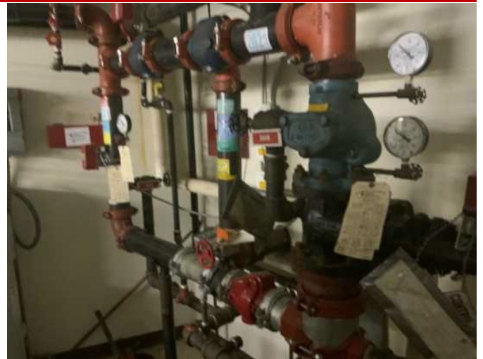
20 - FIRE SUPPRESSION SYSTEM
