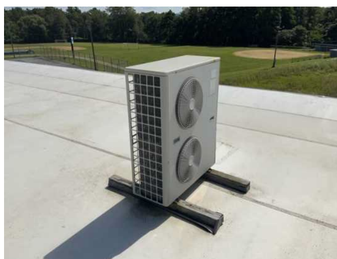
18 - SPLIT SYSTEM DUCTLESS
