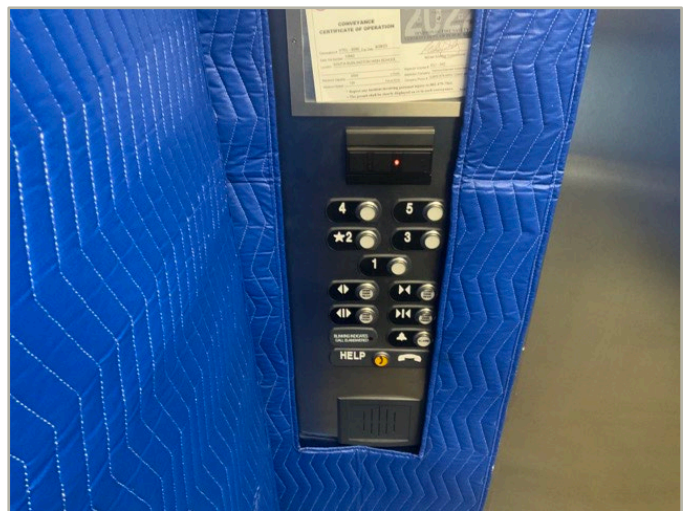
12 - IN-CAB CONTROLS/EMERGENCY CALL PANEL
