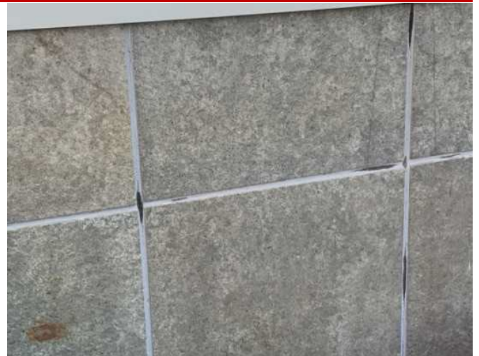
8 - EXTERIOR WALL CAULKING FAILURES
