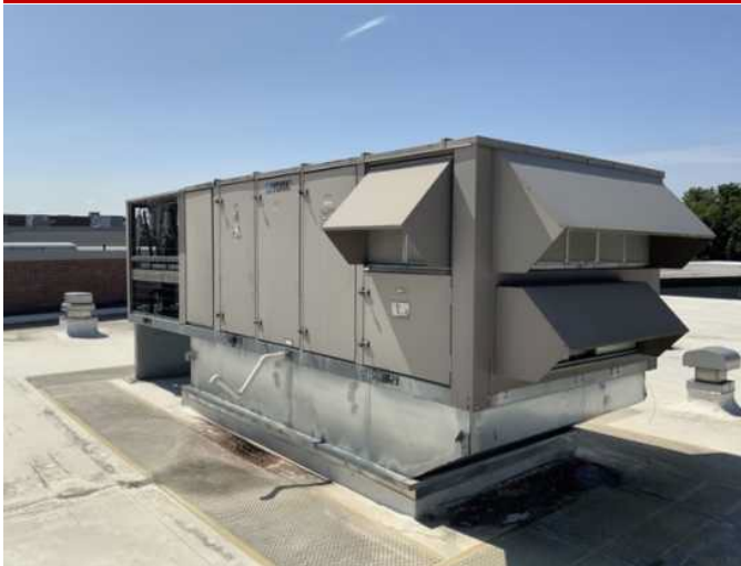
19 - PACKAGED UNIT ON ROOF
