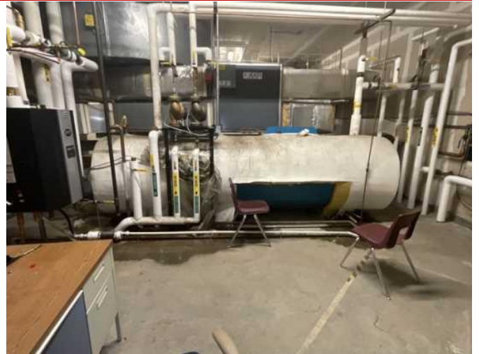
20 - DOMESTIC HOT WATER STORAGE TANK
