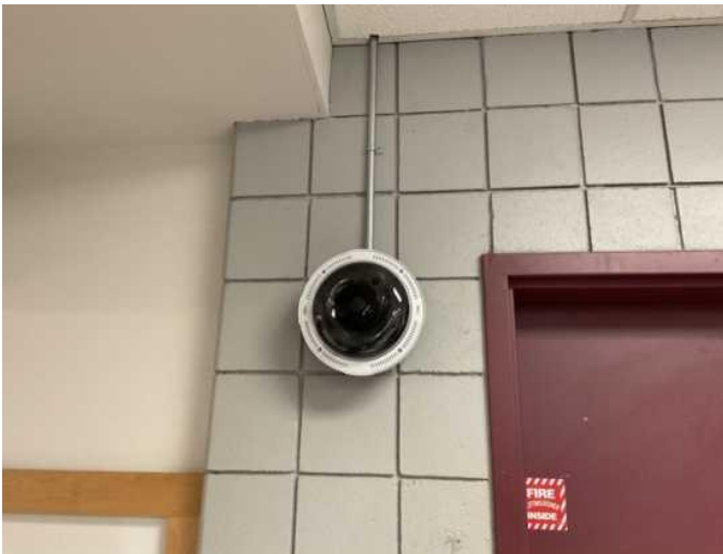
33 - SECURITY SURVEILLANCE CAMERA SYSTEM
