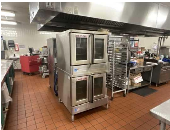
35 - COMMERCIAL FOOD SERVICE EQUIPMENT
