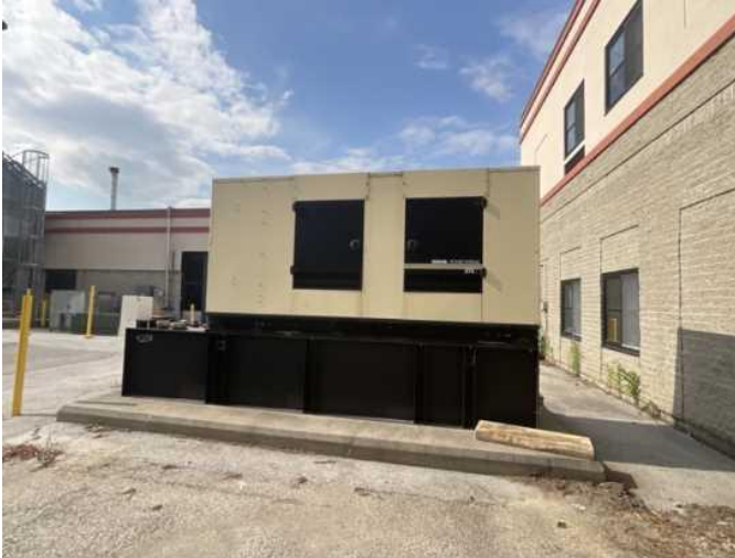
31 - BACKUP DIESEL GENERATOR EQUIPMENT
