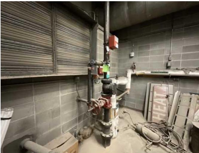
27 - FIRE SUPPRESSION MAIN EQUIPMENT
