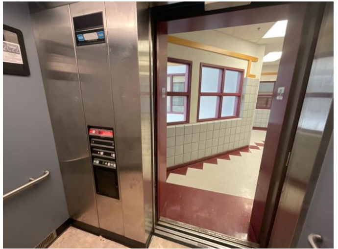
12 - IN-CAB CONTROLS/EMERGENCY CALL PANEL
