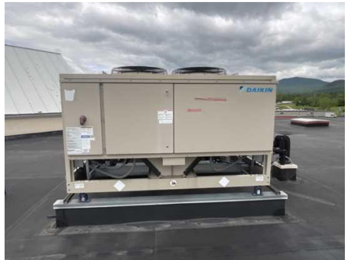
22 - ROOF MOUNTED COOLING TOWER
