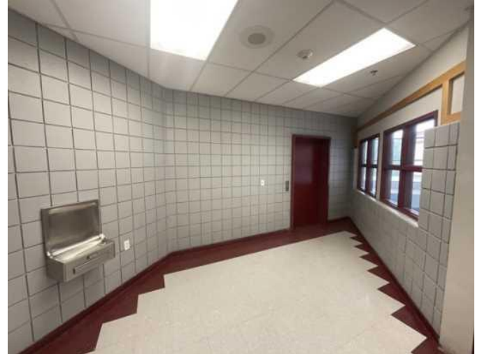
32 - INTERIOR CEILING MOUNTED LIGHTING
