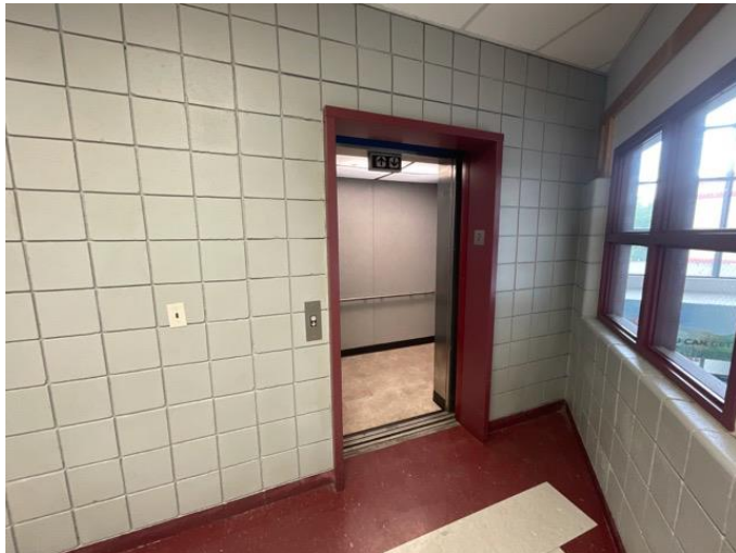
11 - LOBBY VIEW OF CABS, WITH DOORS OPEN
