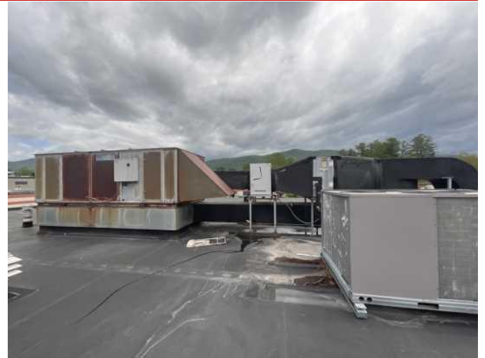
26 - MAKE-UP AIR UNIT
