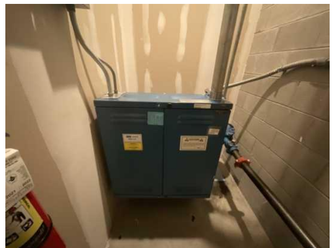
18 - HYDRAULIC ELEVATOR EQUIPMENT ROOM
