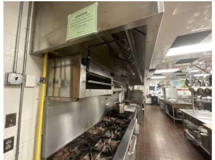
28 - KITCHEN FIRE SUPPRESSION EQUIPMENT
