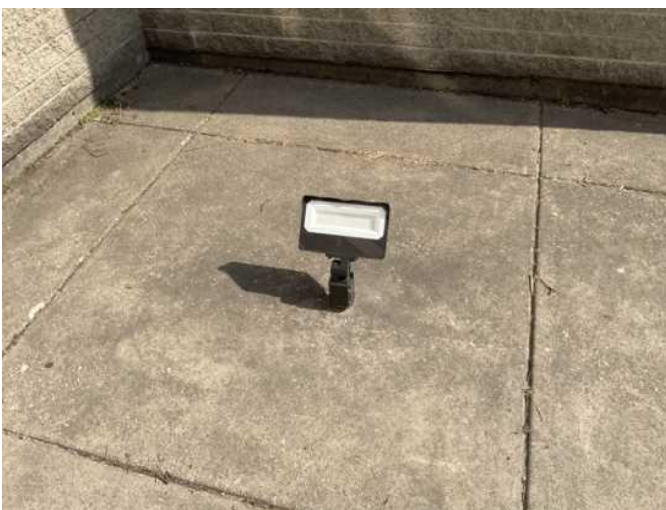
47 - EXTERIOR LED LIGHTING FIXTURE
