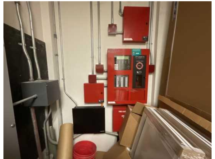
34 - FIRE ALARM SYSTEM PANEL
