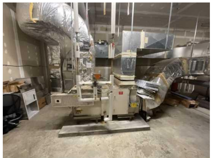
24 - INTERIOR LOCATED AIR HANDLER
