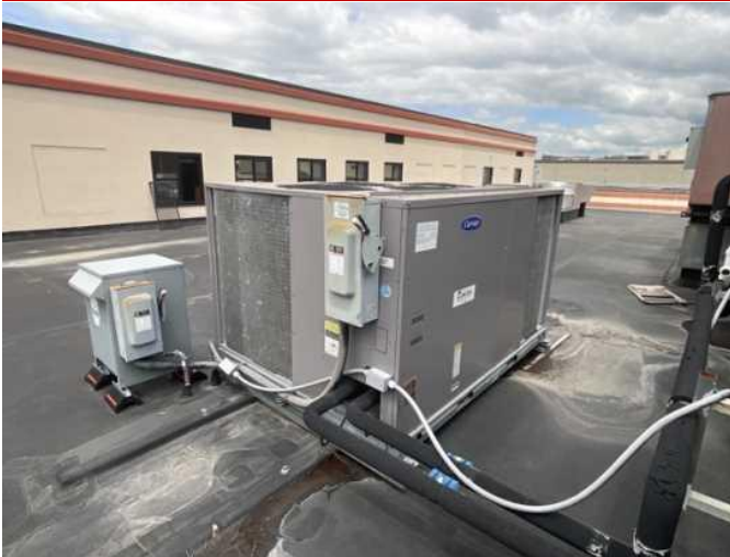
25 - ROOF MOUNTED PACKAGED UNIT
