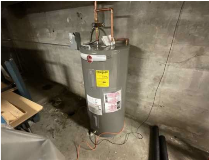
15 - ELECTRIC FUEL WATER HEATER
