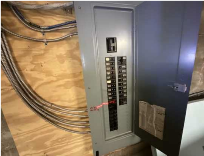
19 - DISTRIBUTION PANEL FOR BUILDING
