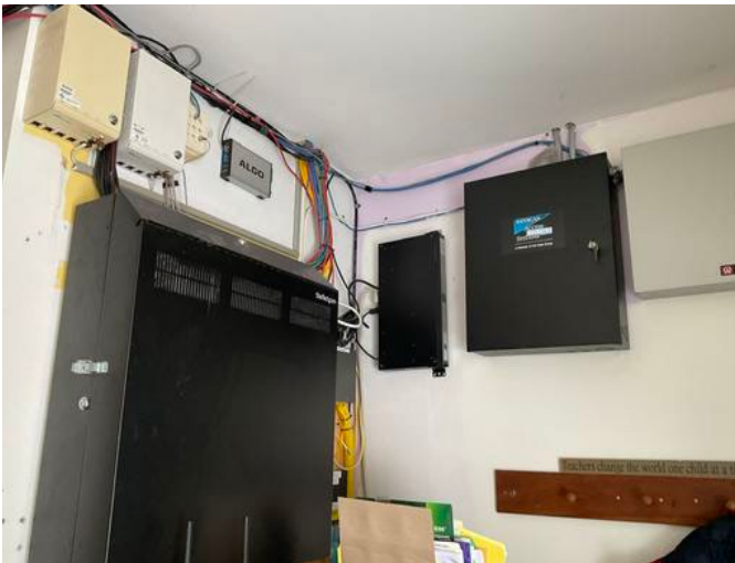
21 - SECURITY AND DATA CENTER
