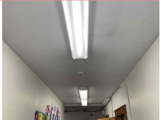
20 - INTERIOR CEILING MOUNTED LIGHTING
