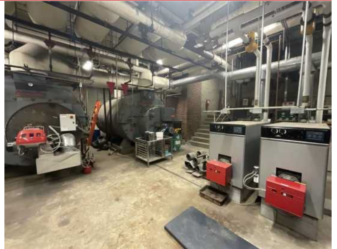
8 - BOILER ROOM OVERVIEW
