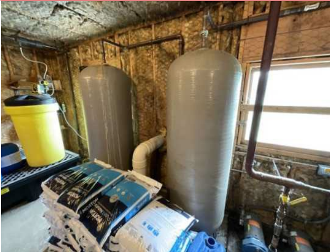
7 - PUMP HOUSE OVERVIEW
