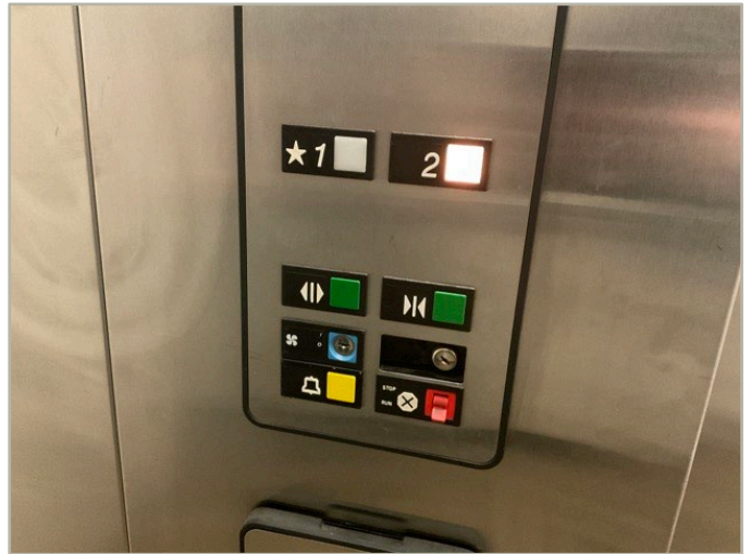
12 - IN-CAB CONTROLS/EMERGENCY CALL PANEL
