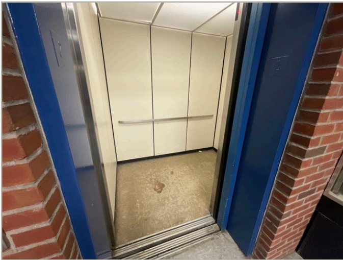
11 - LOBBY VIEW OF CABS, WITH DOORS OPEN
