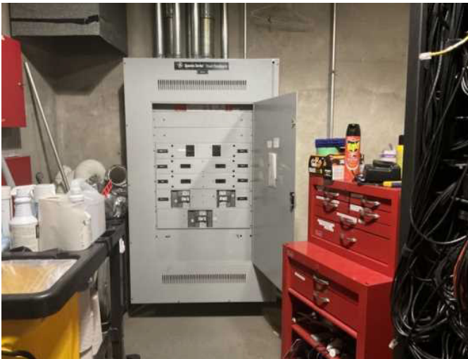
33 - MAIN ELECTRICAL EQUIPMENT
