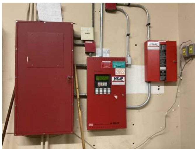
28 - FIRE ALARM PANEL
