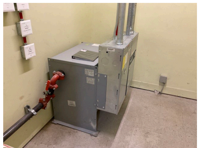
24 - ELEVATOR CONTROLS AND HYDRAULICS
