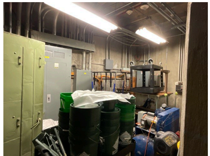
22 - ELECTRICAL ROOM WITH STORAGE
