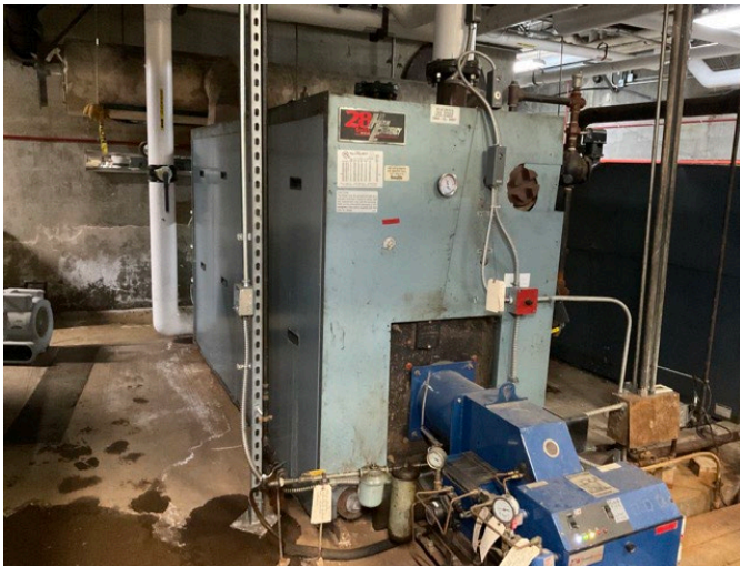
27 - FUEL OIL BOILER OVERVIEW
