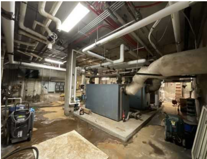
15 - BASEMENT BOILER ROOM OVERVIEW
