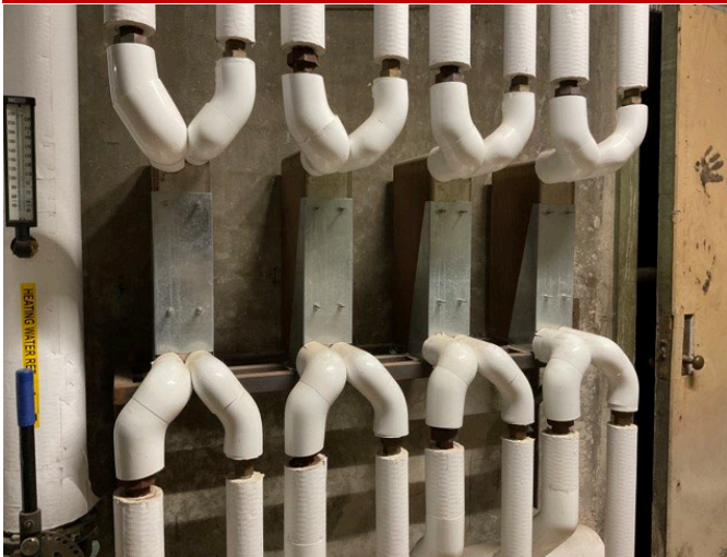
25 - CITY STEAM HEAT EXCHANGE
