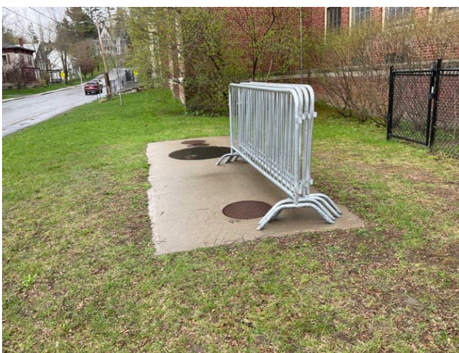
29 - UNDERGROUND STORAGE TANK ACCESS
