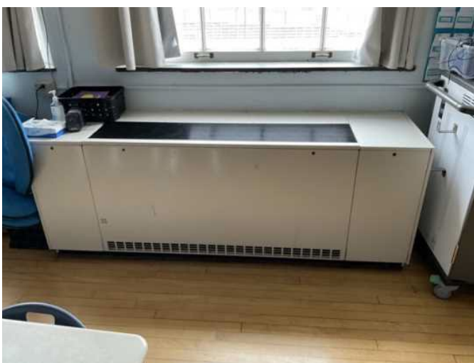
23 - TYPICAL CLASSROOM UNIT VENTILATOR
