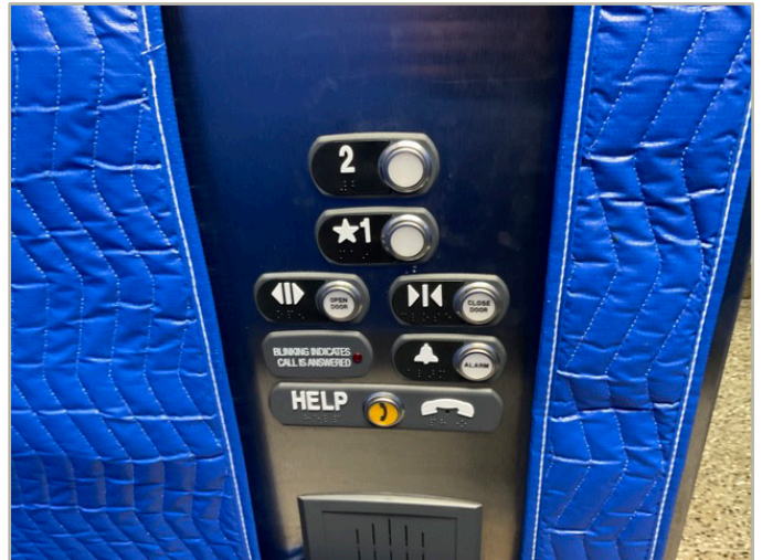
12 - IN-CAB CONTROLS/EMERGENCY CALL PANEL
