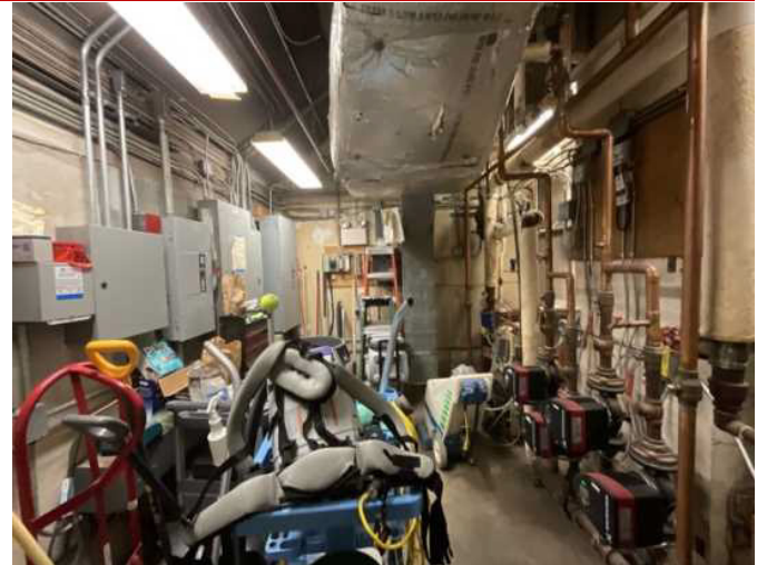
14 - BOILER AND ELECTRICAL ROOM
