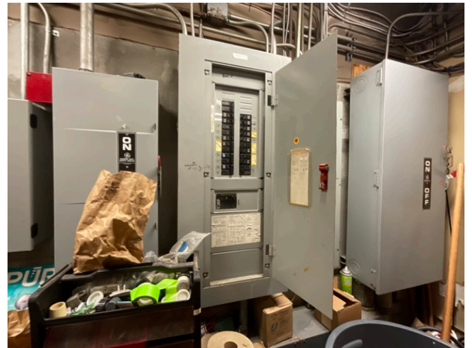
16 - ELECTRICAL SERVICE PANEL OVERVIEW
