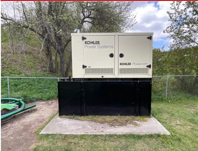
19 - DIESEL BACK-UP GENERATOR
