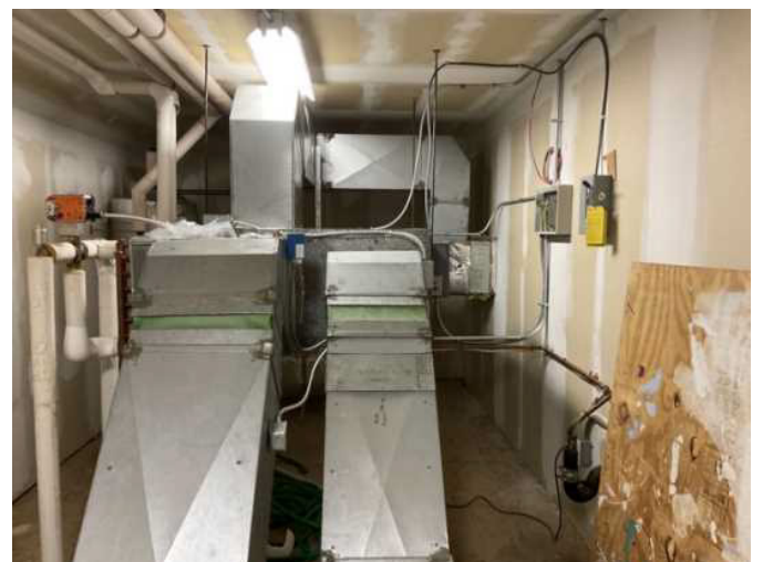
18 - AIR HANDLER OVERVIEW PHOTO
