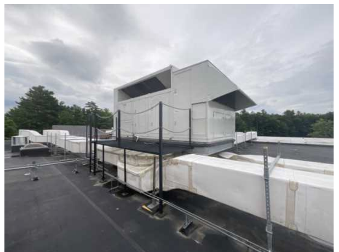
12 - RTU PACKAGED UNIT
