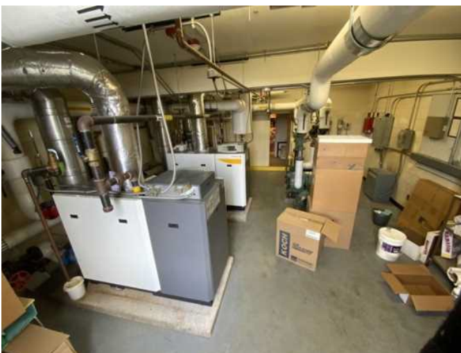
17 - PHOTO OF THE HVAC BOILERS
