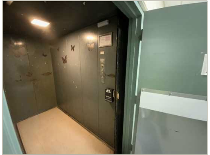
14 - IN-CAB CONTROLS/EMERGENCY CALL PANEL
