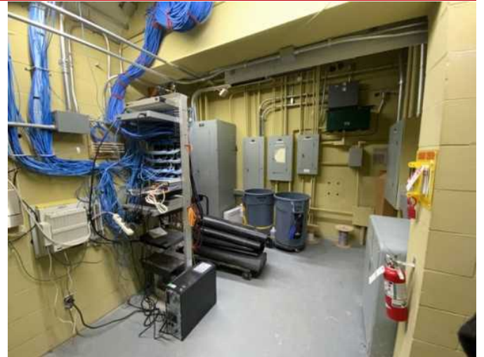
20 - PHOTO OF ELECTRICAL DISTRIBUTION AREA
