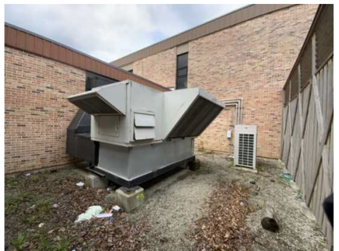
18 - PHOTO OF AN EXTERIOR AIR HANDLER
