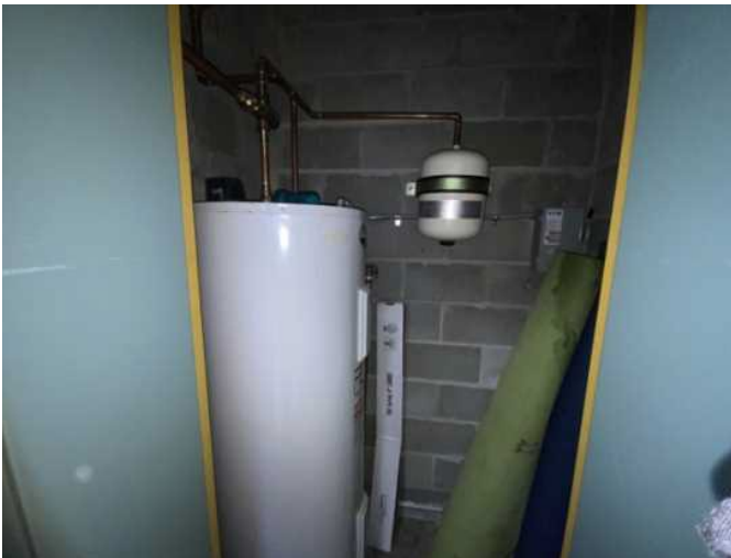
21 - PHOTO OF A WATER HEATER
