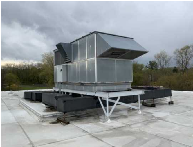
19 - PHOTO OF AN AIR HANDLER
