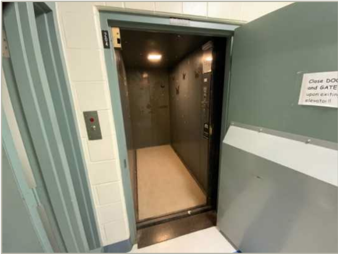
13 - LOBBY VIEW OF CABS, WITH DOORS OPEN
