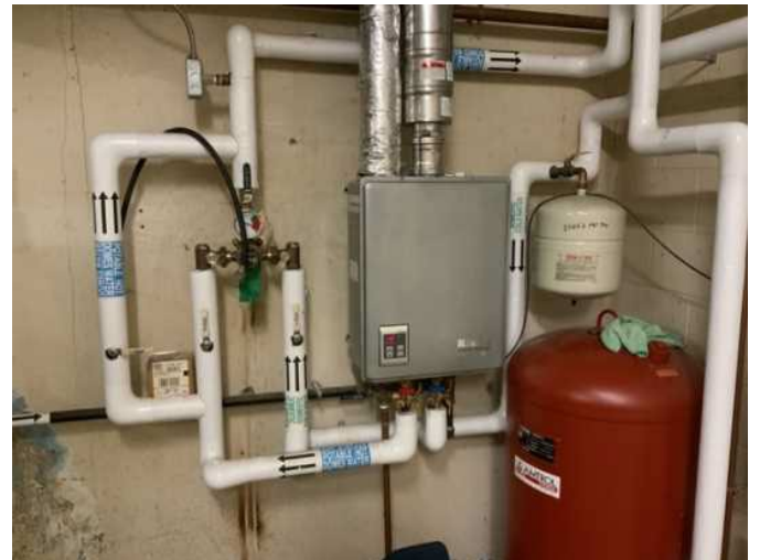
22 - PHOTO OF A WATER HEATER
