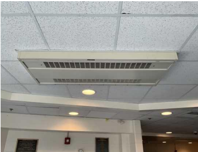
39 - CEILING MOUNTED FAN COIL UNIT
