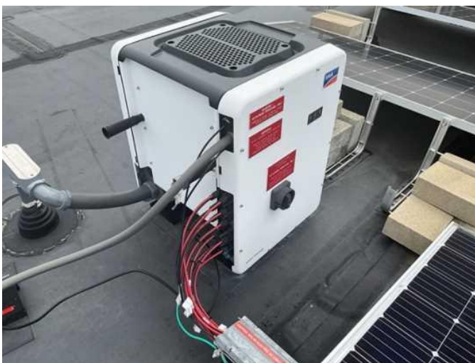
53 - ROOFTOP SOLAR POWER INVERTER
