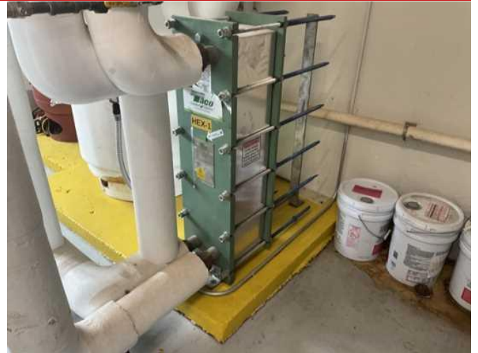
38 - PLATE AND FRAME HEAT EXCHANGER
