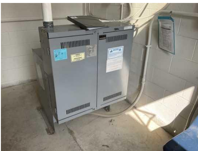
23 - HYDRAULIC ELEVATOR CONTROLs
