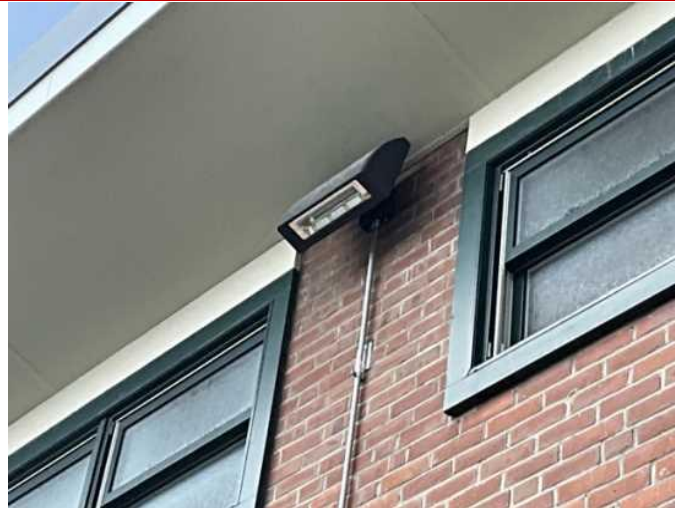
56 - WALL MOUNTED EXTERIOR LIGHTING
