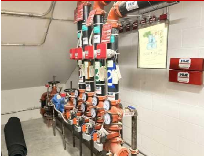
49 - FIRE RISER PIPING AND VALVES
