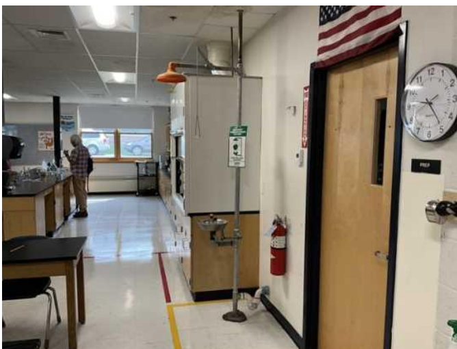
35 - EMERGENCY EYEWASH AND SHOWER
