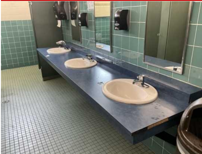
31 - RESTROOM DROP IN STYLE SINKS
