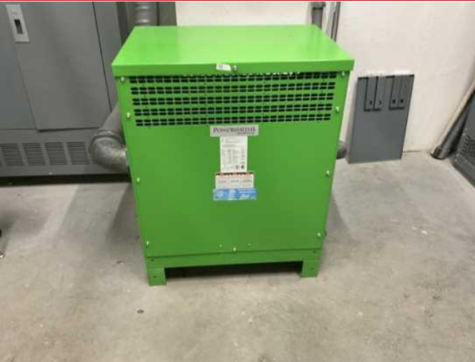
55 - SECONDARY TRANSFORMER DRY TYPE
