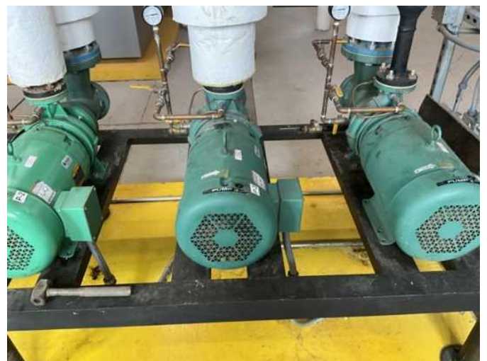
42 - HEATING WATER CIRCULATION PUMPS
