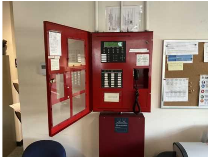
58 - FIRE ALARM PANEL MAIN OFFICE
