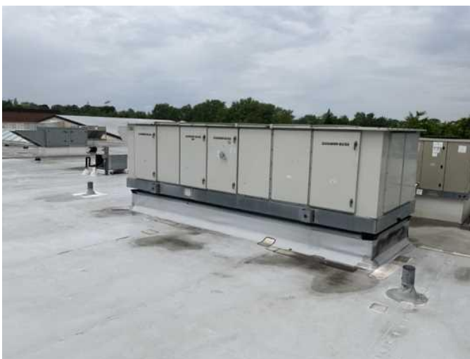
47 - ROOF TOP AIR HANDLER
