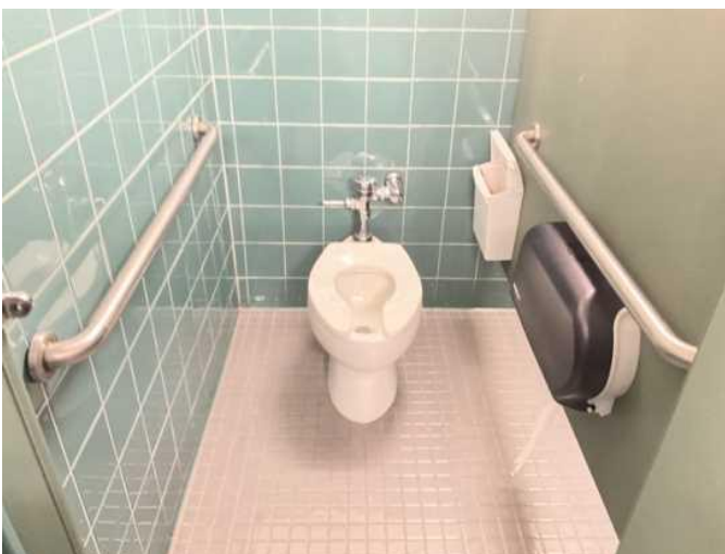
29 - COMMERCIAL WATER CLOSET TOILET
