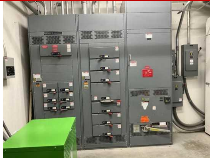
50 - SWITCHBOARD WITH MAIN DISCONNECT
