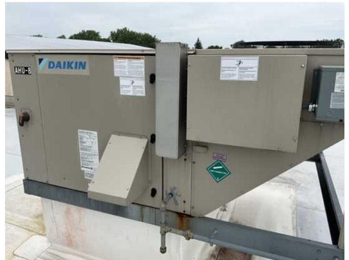
46 - ROOF TOP PACKAGED UNIT
