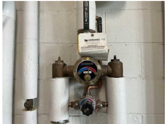
34 - HOT WATER MIXING VALVE
