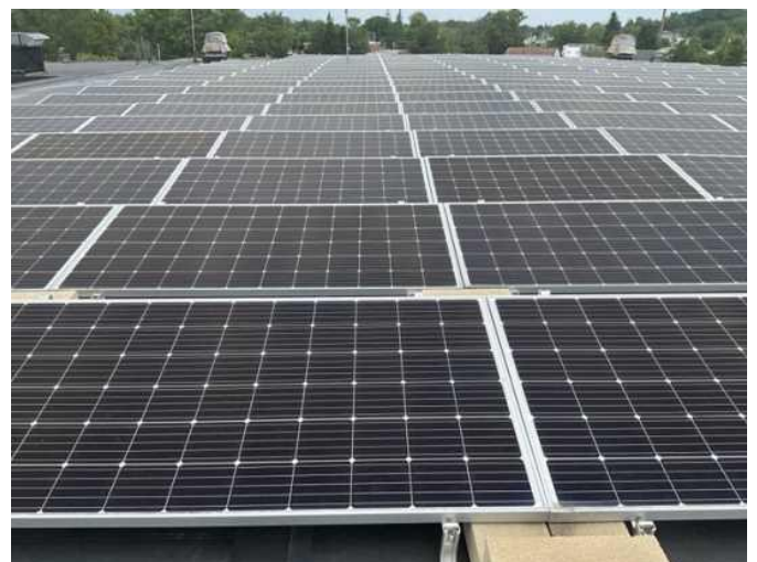
54 - SOLAR POWER PHOTOVOLTAIC PANELS
