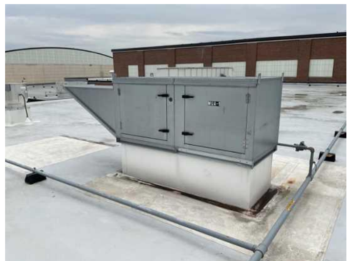
48 - MAKE-UP AIR UNIT
