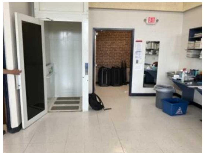
22 - HANDICAP ELEVATOR- TWO FLOORS
