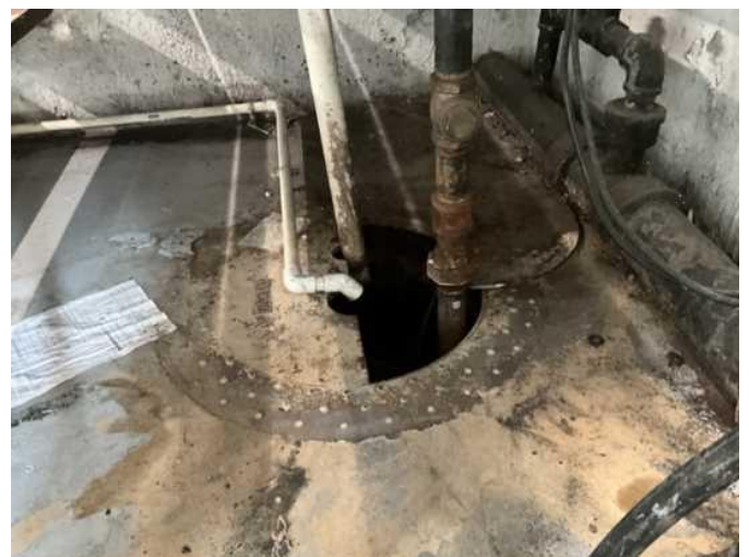
36 - BOILER ROOM SUMP PUMP
