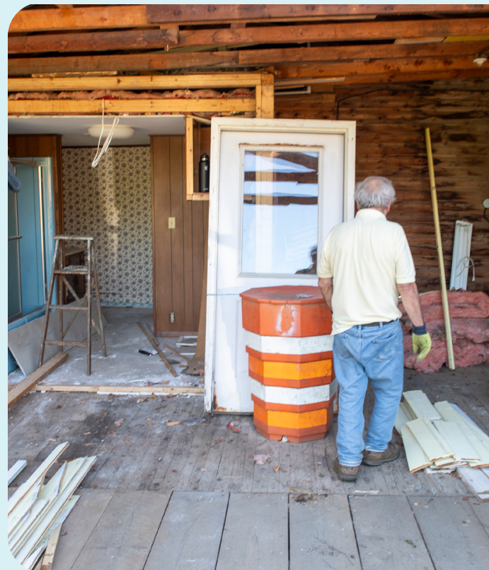
A home affected by flood-induced erosion was bought out.
