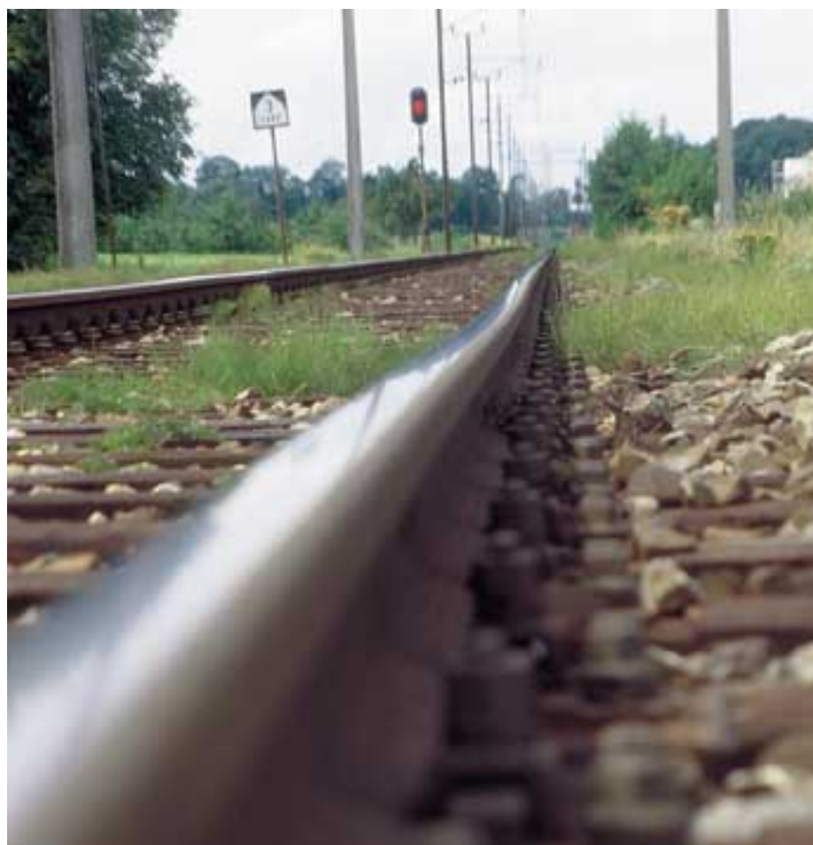
Plants are excellent indicators of the state of the soil. The rich growth of horsetail in the picture shows that the ground in this area is damp and therefore unstable. Here, the result has been track subsidence.
