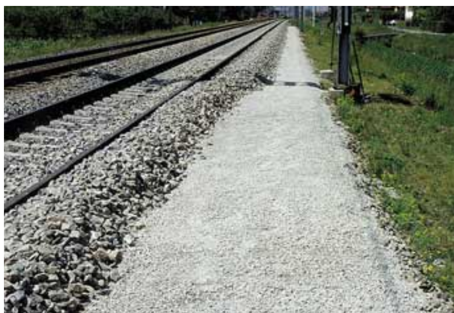
The extent to which ballast must be free of vegetation depends above all on the number of trains and their speeds.
