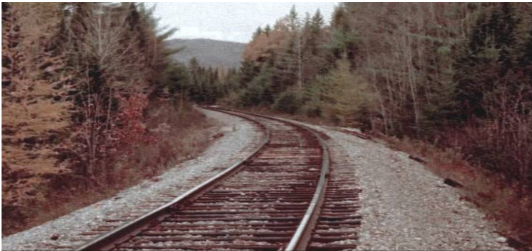
Figure 9: Typical “extensive treatment” track condition
