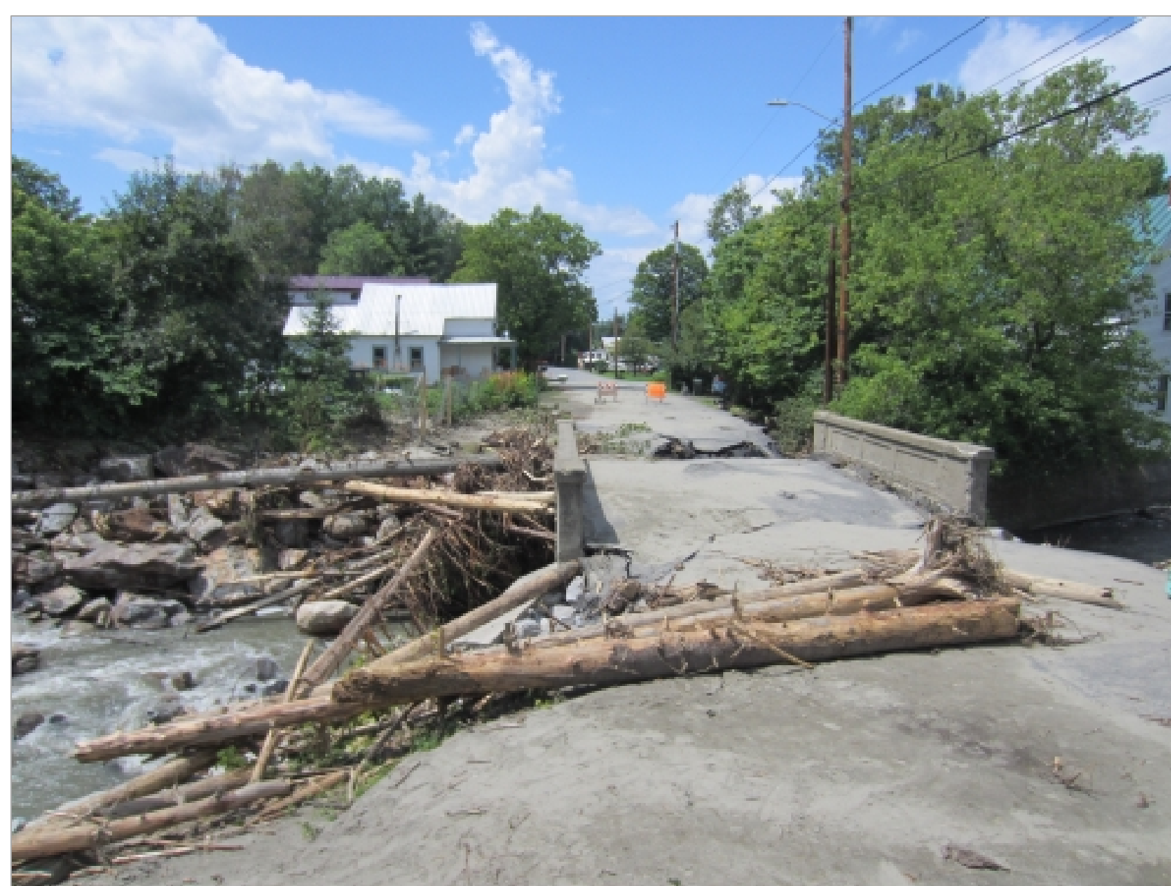
Damage caused by debris blockage of a crossing structure
