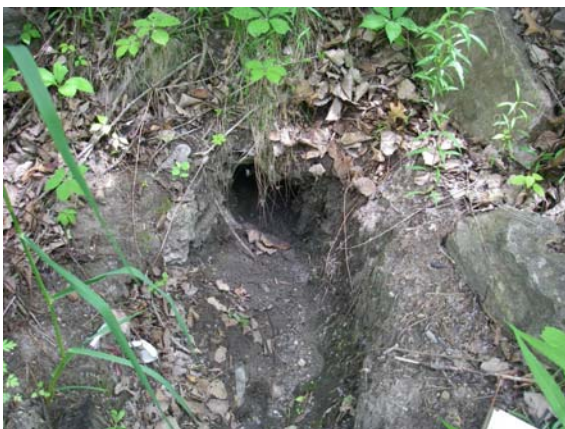
Outfall 51A: 24" RCP
