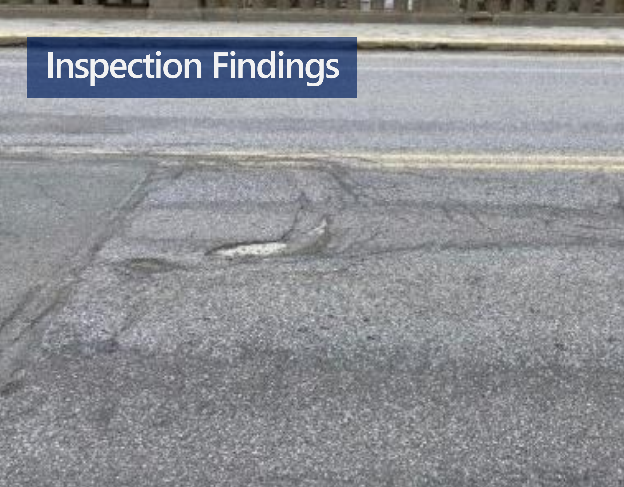
Depression Cracking and Exposed Deck Surface
