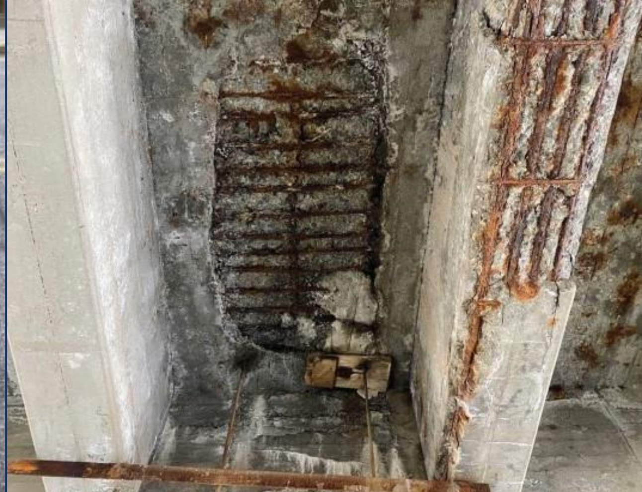
Probable Full-Depth Deck Hole in Bay 4 with Severe Concrete Spalling and Corroded Reinforcing
