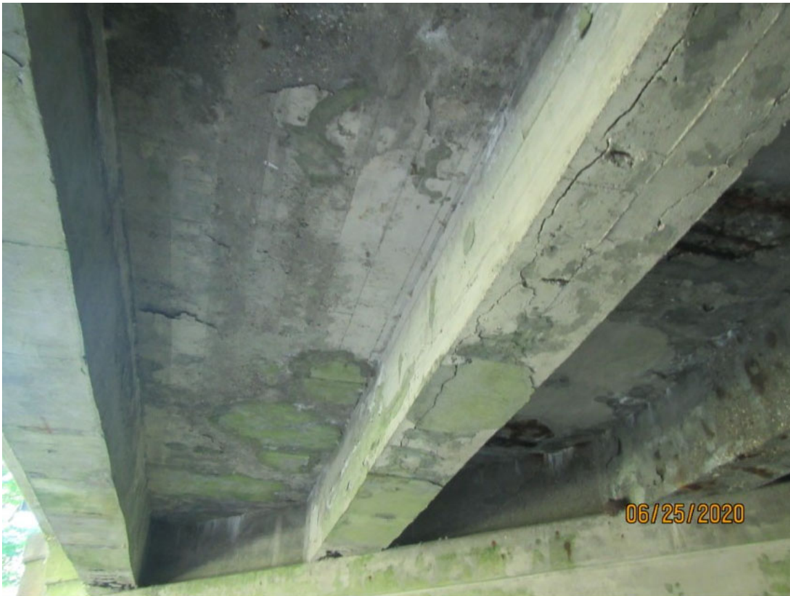
Picture 9: T-beam deterioration
