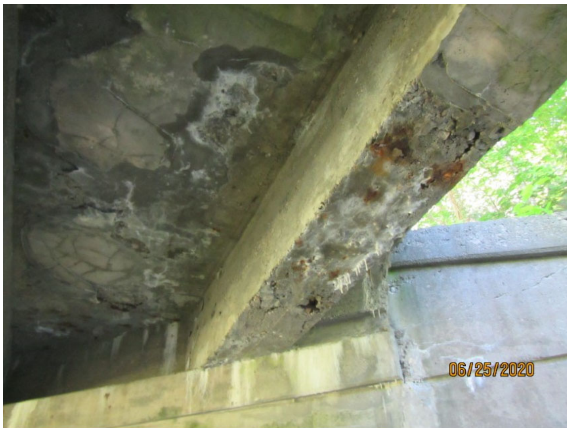
Picture 11: T-beam deterioration
