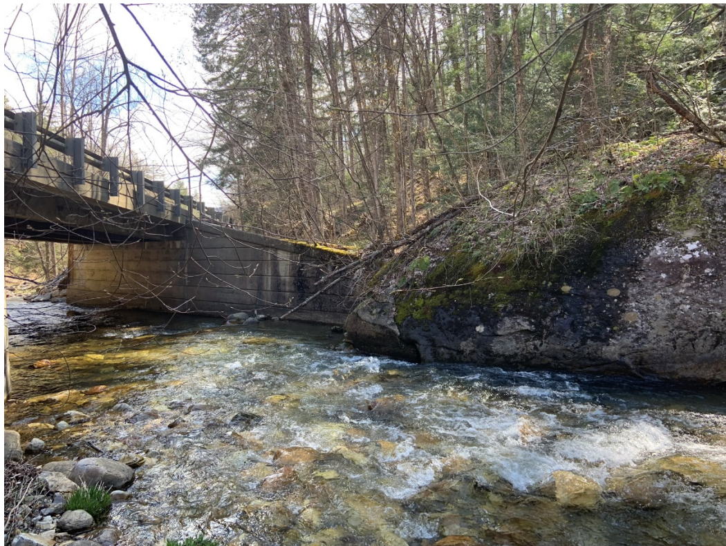
Figure 3.5: Large boulder present upstream of bridge, note presence of cobbles and boulders in streambed.
