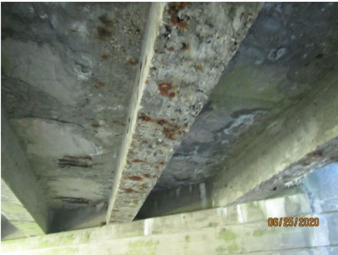
Picture 10: T-beam deterioration
