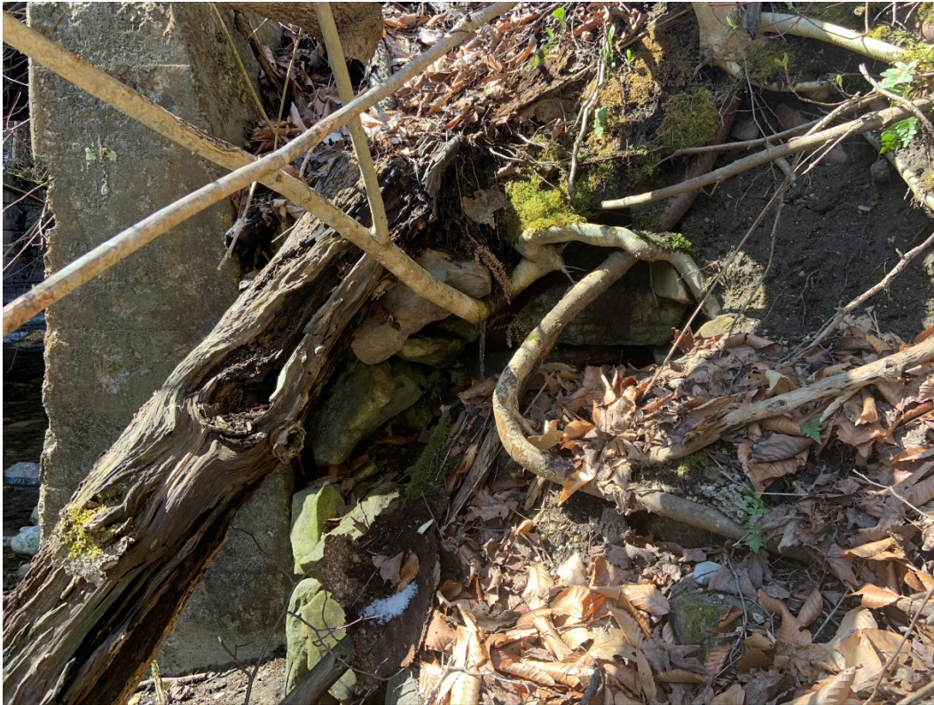
Figure 3.4 Western downstream wingwall of bridge, note voids present within cobble and sand backfill.
