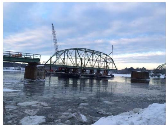
A Detailed Demolition Plan will be Followed by R&R Crews to Ensure Bridge Stability and Safety
