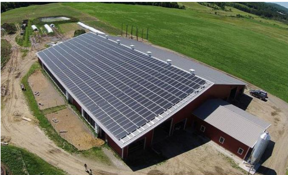
181 KW ROOF TOP SOLAR ARRAY ON GOAT BARN AT AYERS BROOK GOAT DAIRY IN RANDOLPH
