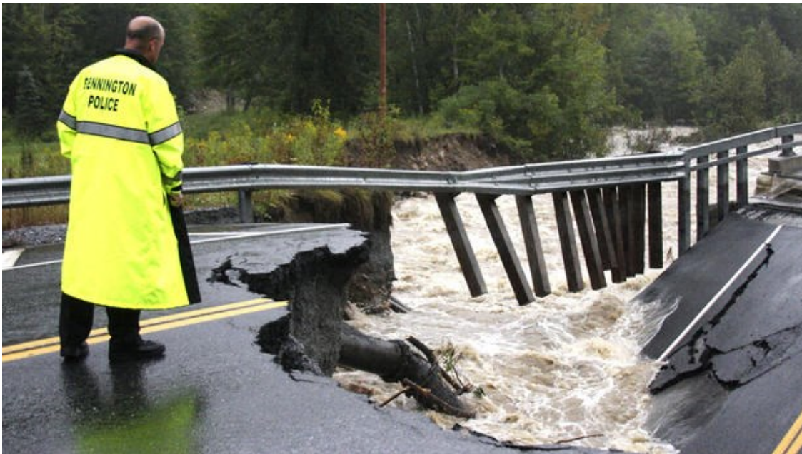
Preventative actions and emergency response preparedness can help mitigate the impact of flood events such as the one pictured above, which compromised a transportation corridor in Bennington (photo from cbsnews.com).
