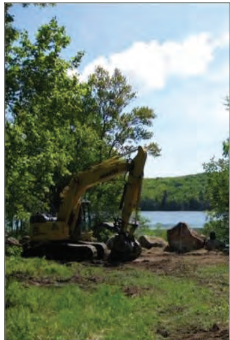
Recent work at the shore of Sucker Pond reduced erosion and improved water quality and public access (US Forest Service photo).
