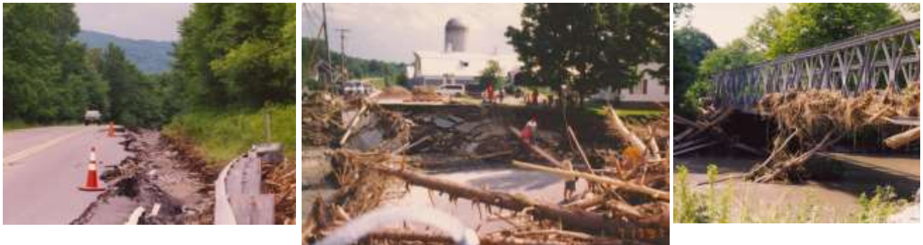
Photos of flood damage from the 1997 Montgomery Flood
