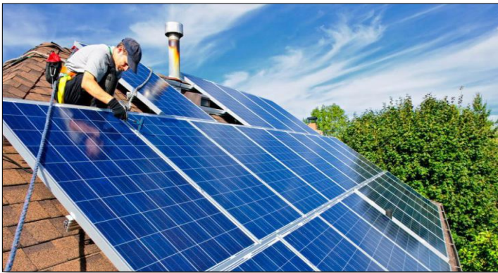
Courtesy: Rob Stubbins Solar Energy
