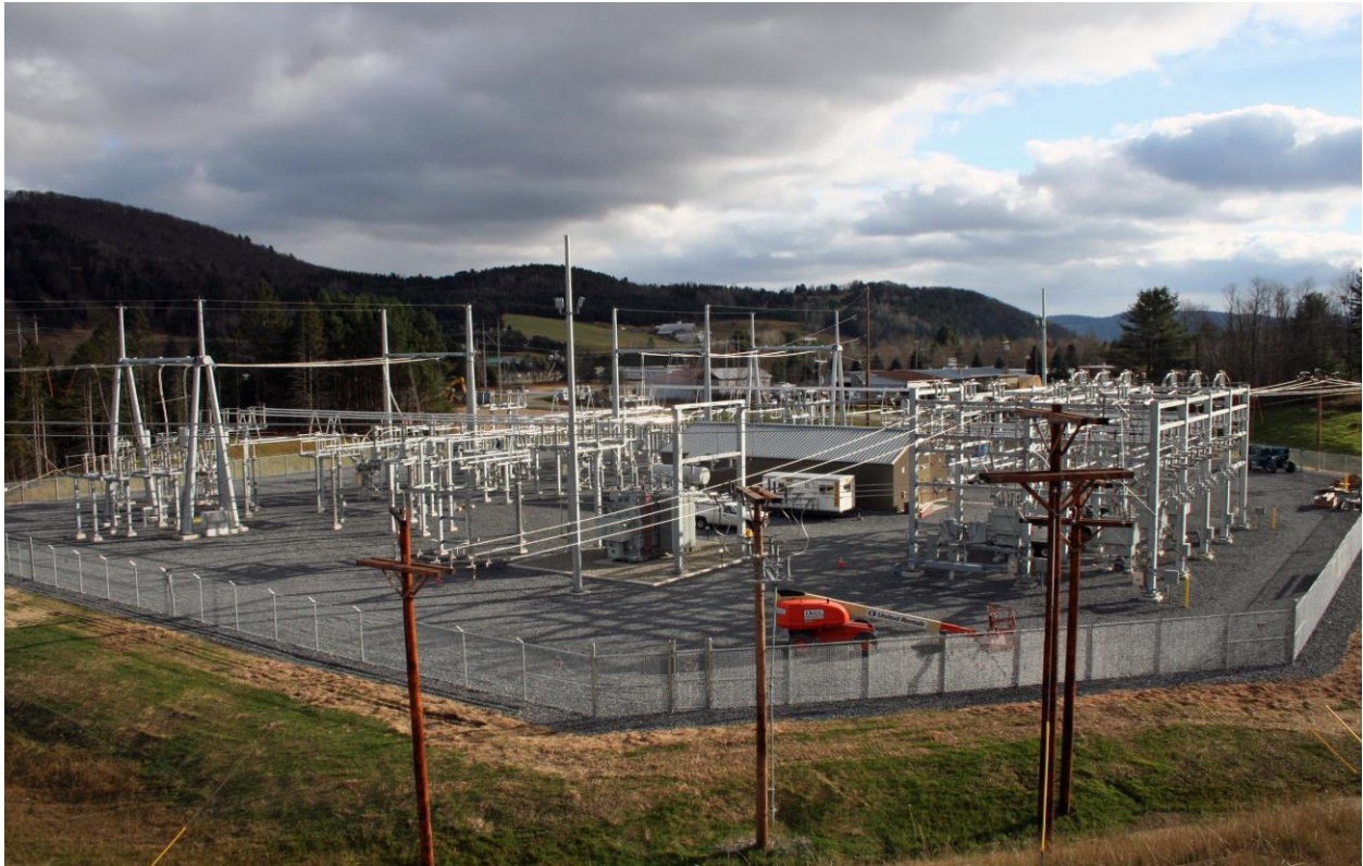
New Sub-Station, Lyndonville Electric Department
