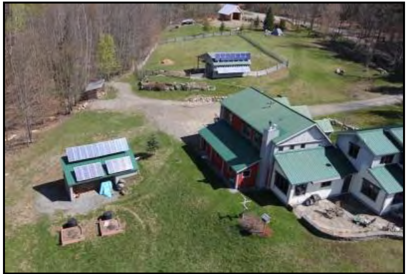
Photo: Solar panel installations in Lamoille County, courtesy of Over and Above Aerial Photography
