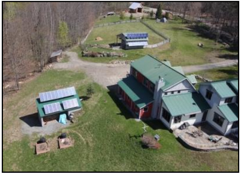
Solar panel installations in Lamoille County Photo by: Over and Above Aerial Photography
