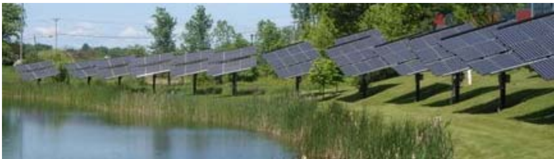
NRG Systems Solar Tracker Array, photo by Carrie Fenn
