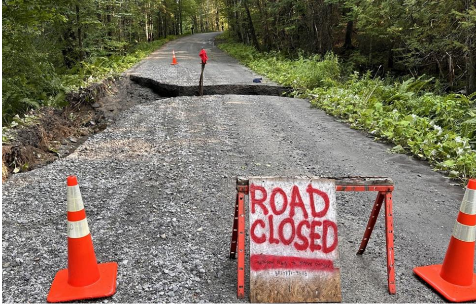
Figure 14 Road washout Photo by Mary Orth
