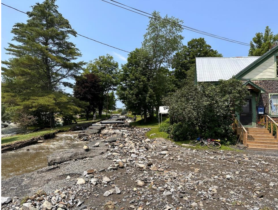
Figure 13 Road washed-out in front of Adamant Co-op July 2023 Photo by Mary Orth
