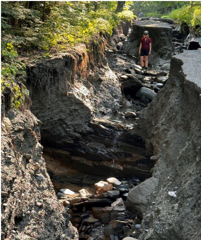
Figure 17 Bliss Pond Road wash-out July 2023 Photo by Mary Orth
