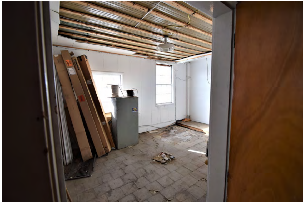
Photo 44: Building #4, view shows a second of the three offices in the lakeside pavilion; note the bead-board ceiling under the acoustic tiles
