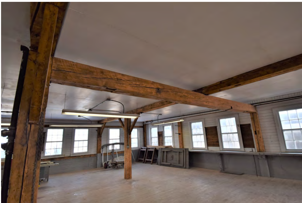
Photo 41: Building #4, view shows second floor header beam in lieu of post in this area
