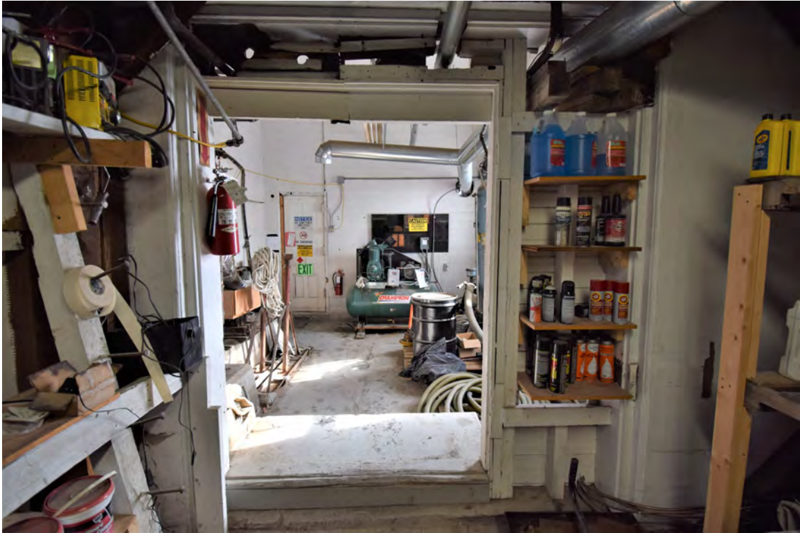
Photo 35: Building #4, view looking southeast from main block first floor into the lakeside pavilion.
