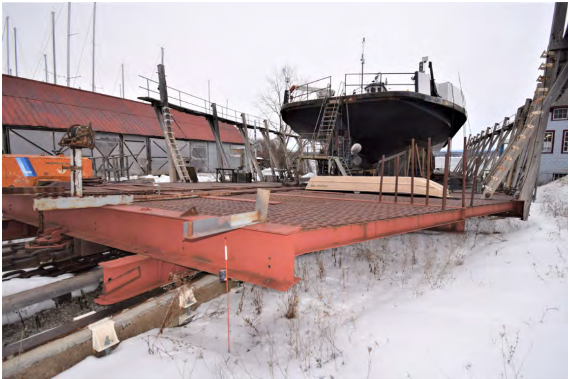
Photo 70: Structure #12, view looking southeast, shows steel framed cradle with metal grate floor and wood catwalk
