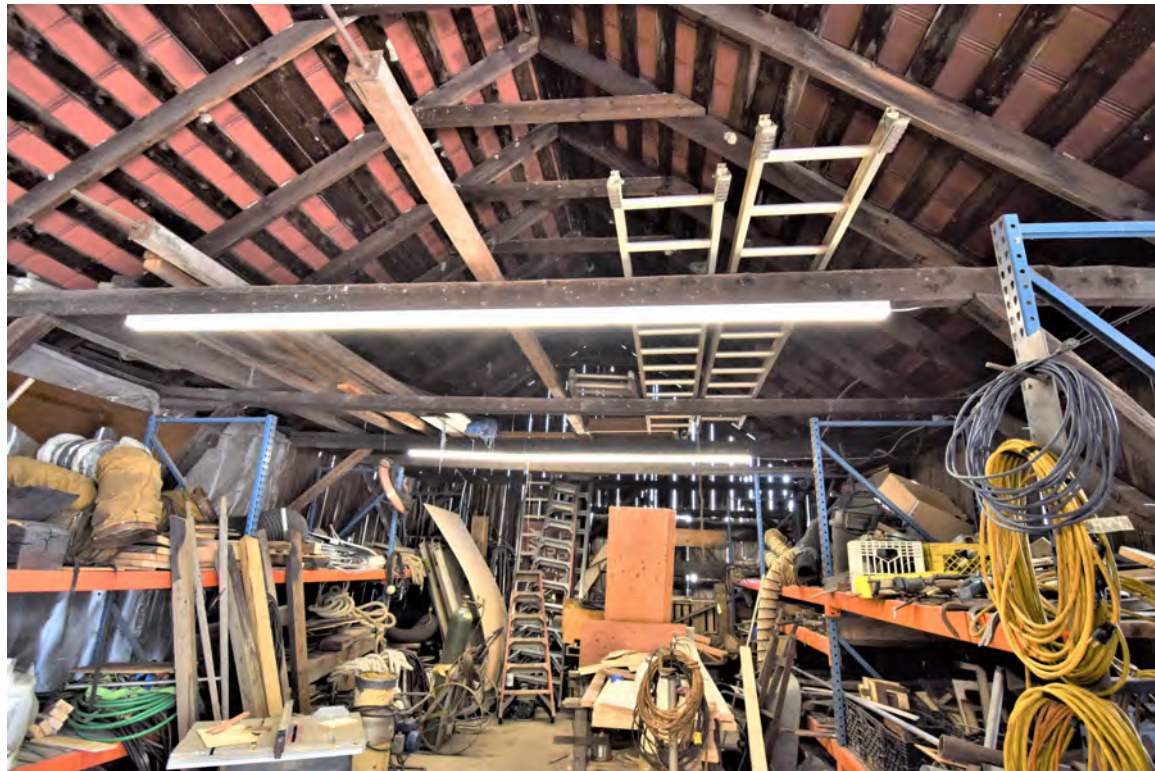
Photo 64: Building #10, view looking southeast, shows interior conditions
