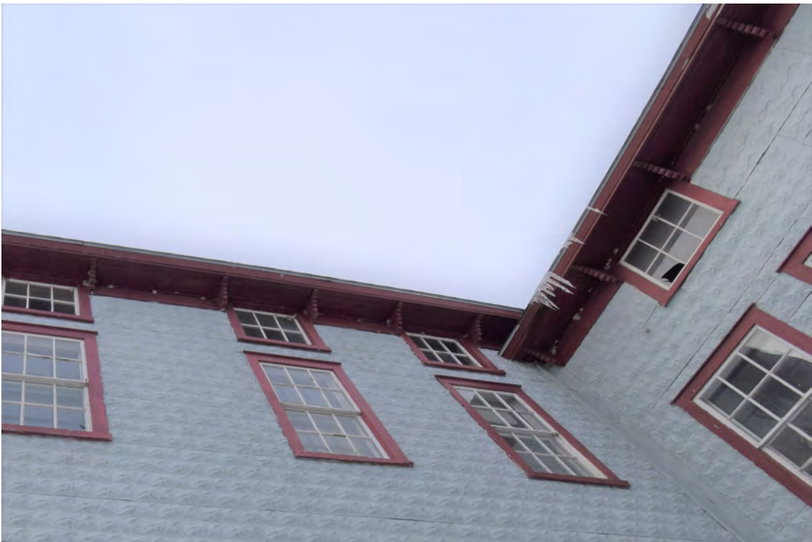
Photo 24: Building #4, view looking north, shows eaves at fiberglass shop / main block intersection
