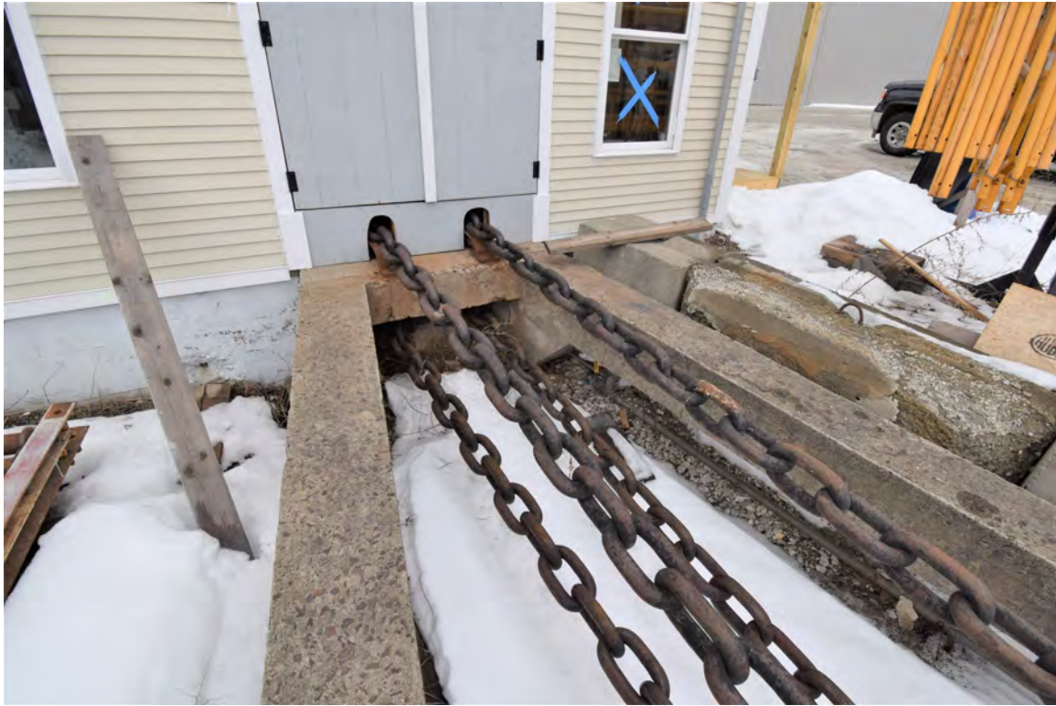
Photo 69: Structure #12, view looking northwest, shows haul chains passing through wall of marine railway powerhouse (resource #5)
