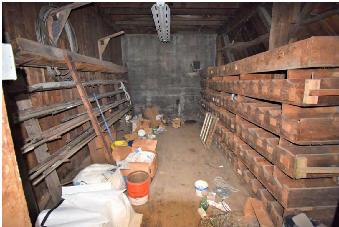
Photo 27: Building #4, view looking northwest into one of three storerooms behind the machine shop.
