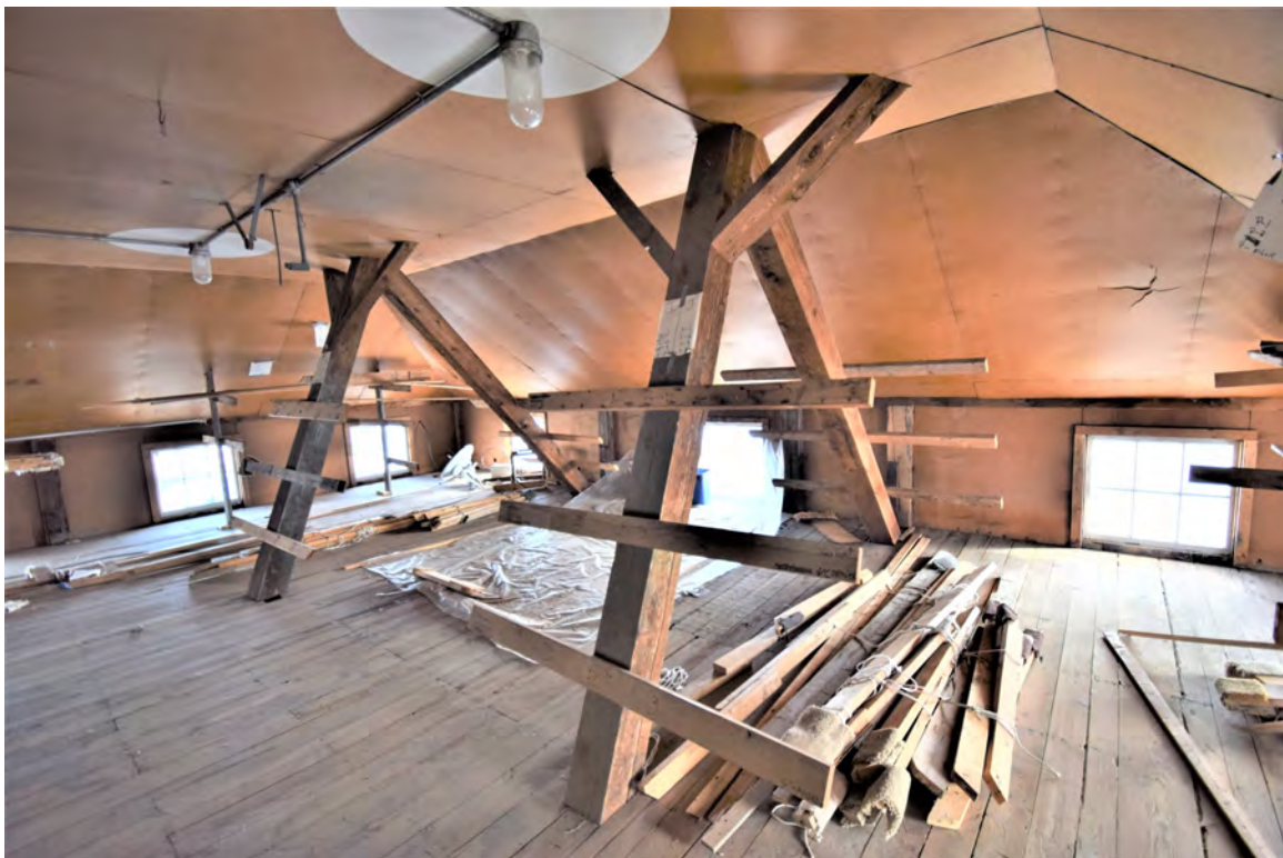
Photo 52: Building #4, view shows detail of timber diagonals in lakeside pavilion 3rd floor
