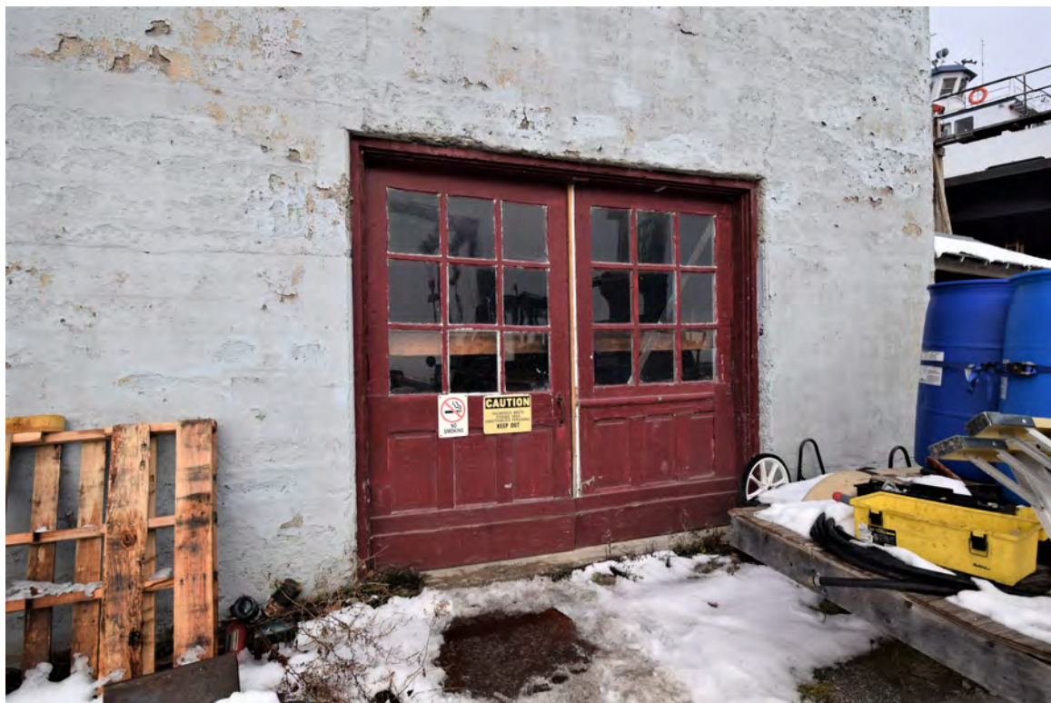
Photo 22: Building #4, view looking north, shows paired exterior doors accessing lake-facing elevation of projection
