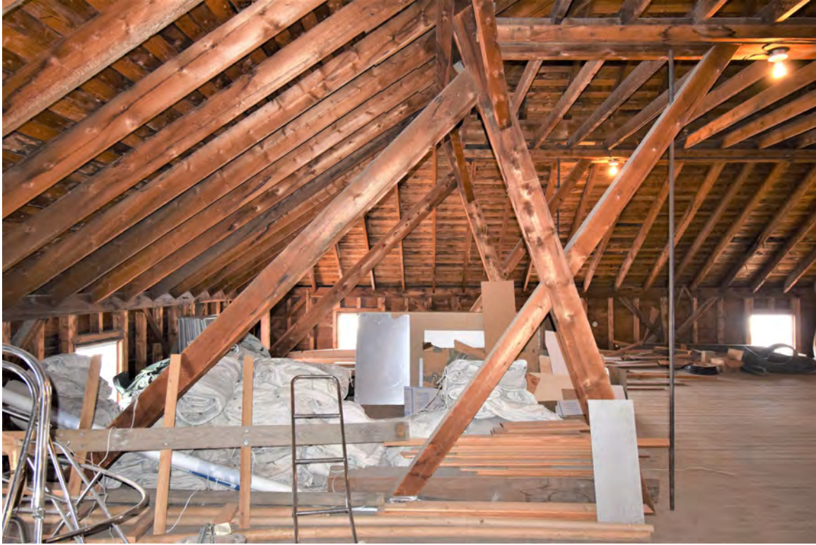
Photo 47: Building #4, view shows roof timberframe support and rafters detail in main block third floor
