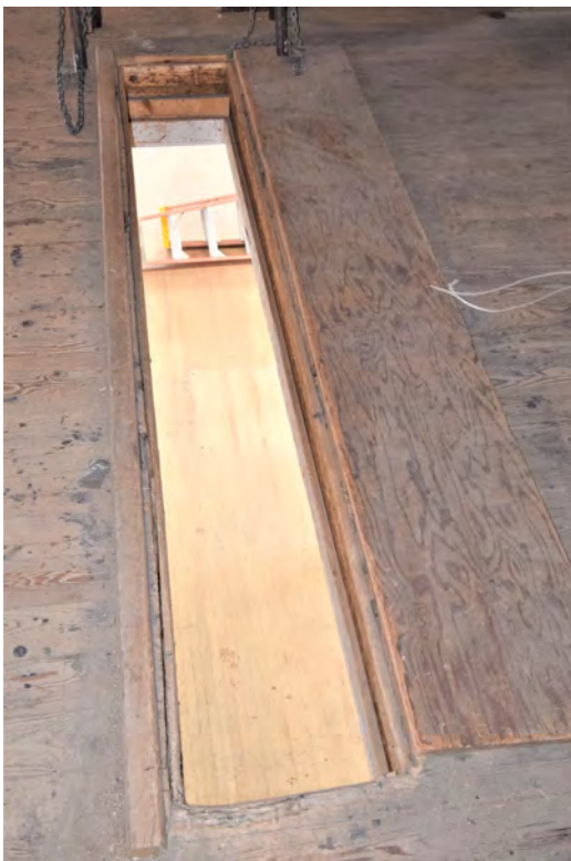
Photo 48: Building #4, view shows original slot in for moving lumber between the main block 2nd and 3rd floors
