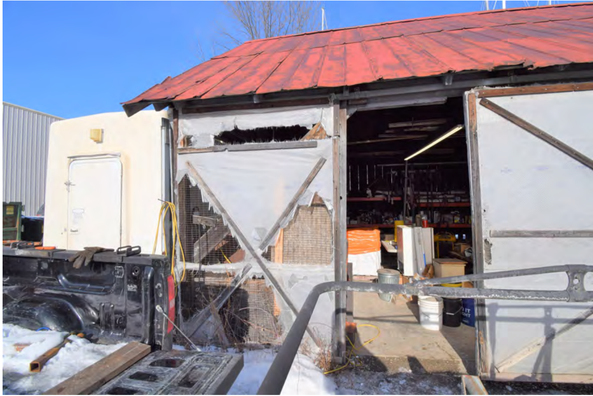
Photo 63: Building #10, view looking northeast, shows concrete slab floor and deteriorating, replacement sliding doors
