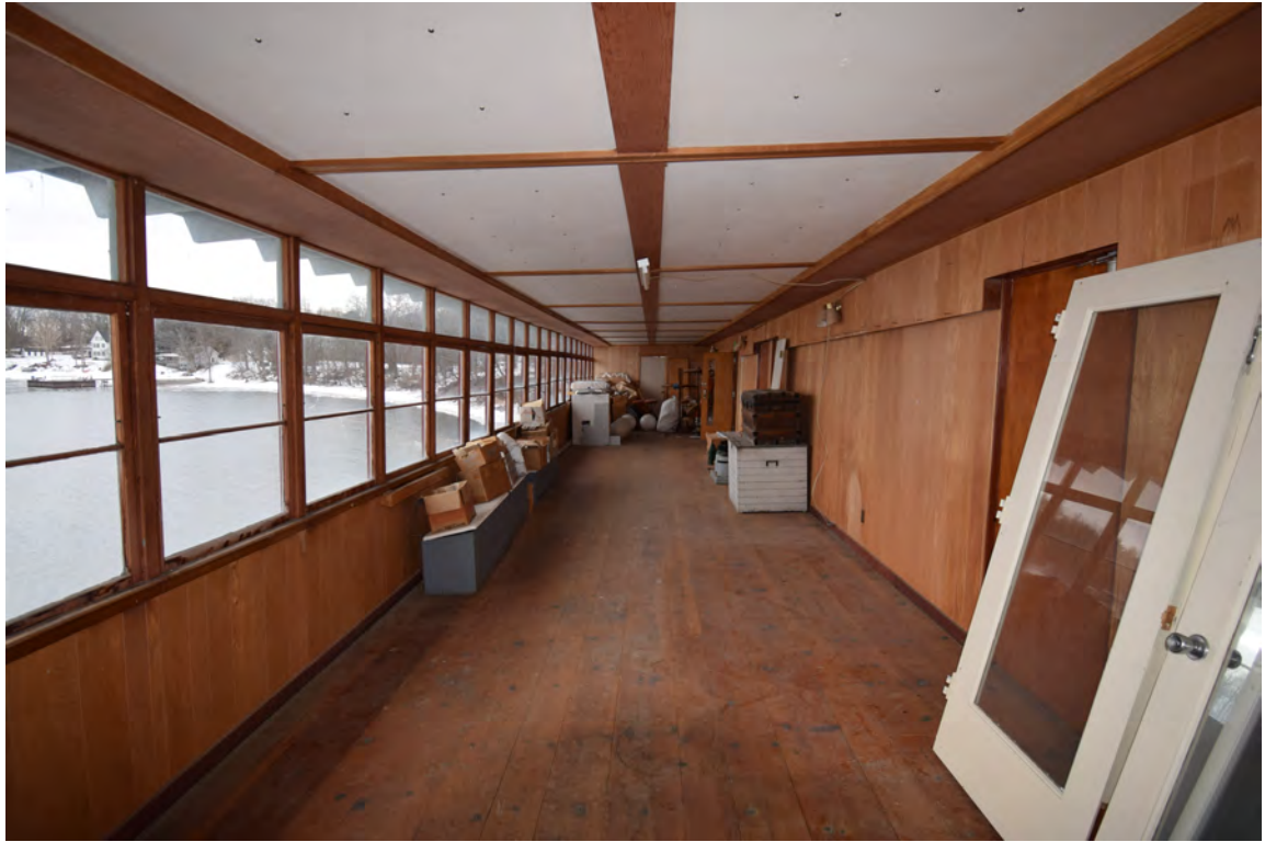
Photo 7: Building #1, view shows second floor porch interior conditions
