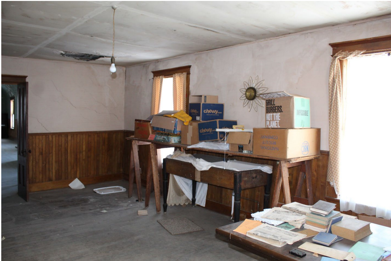
Vermont_LamoilleCounty_GihonValleyGrangeHall_0014: Interior, second floor showing the former kitchen space. Camera facing northeast.
