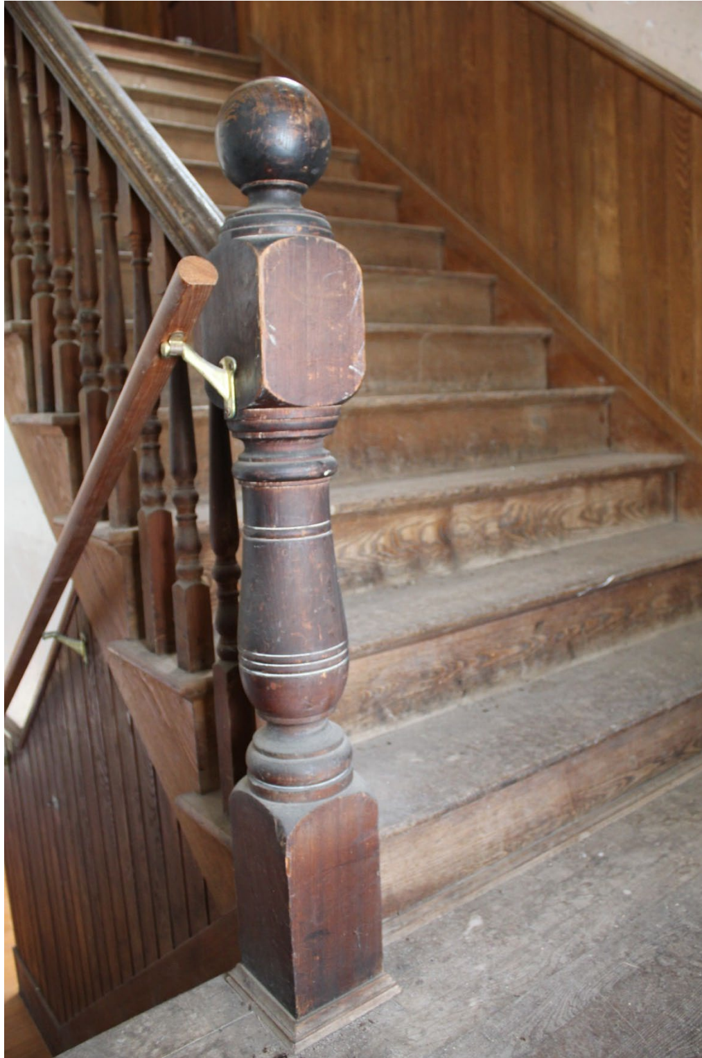
Vermont_LamoilleCounty_GihonValleyGrangeHall_0012: Interior, second floor detail photo of the staircase's newel post. Camera facing northeast.
