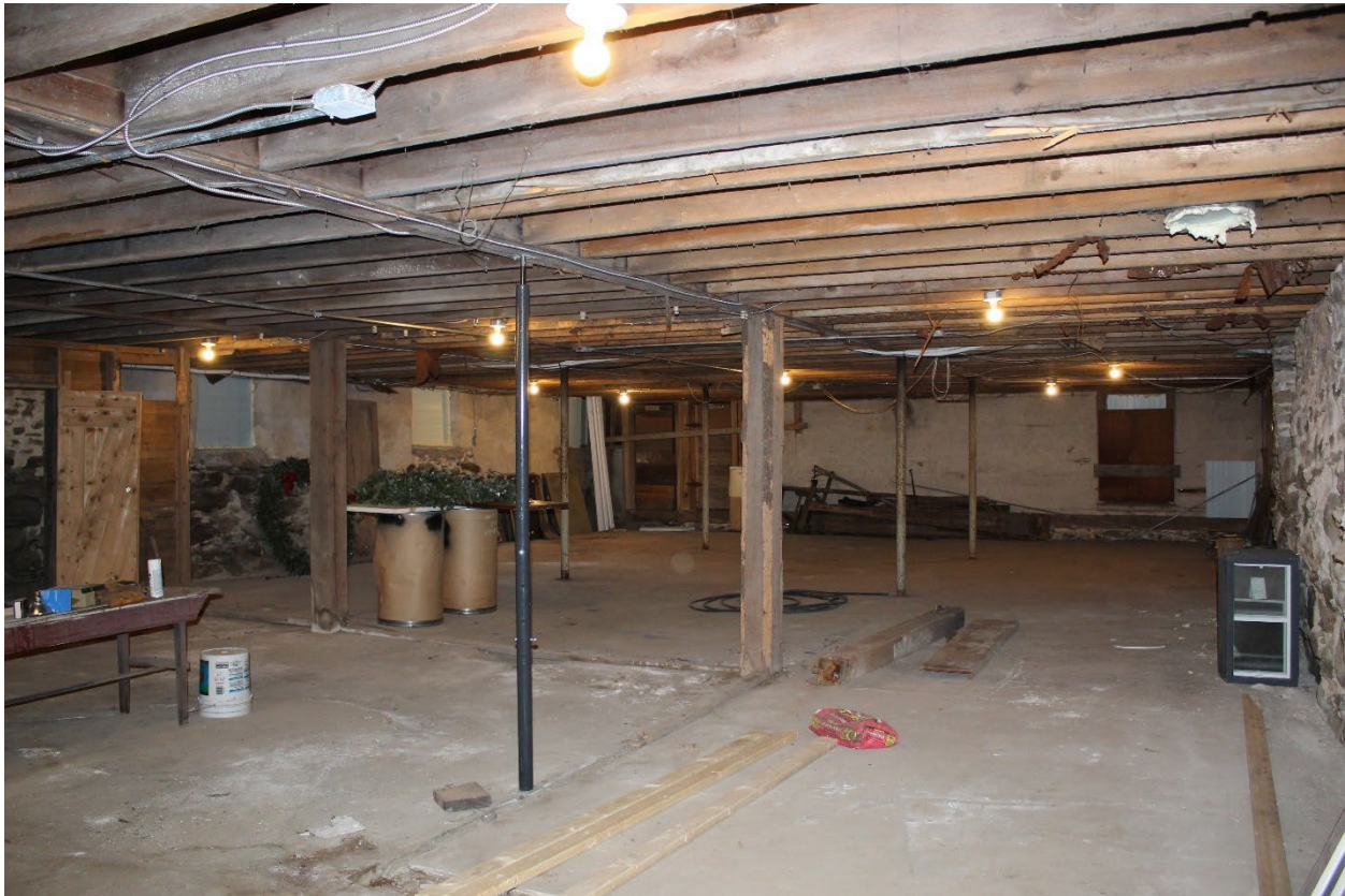
Vermont_LamoilleCounty_GihonValleyGrangeHall_0006: Interior, basement showing the stone foundation which has been reinforced with concrete. Camera facing northwest.
