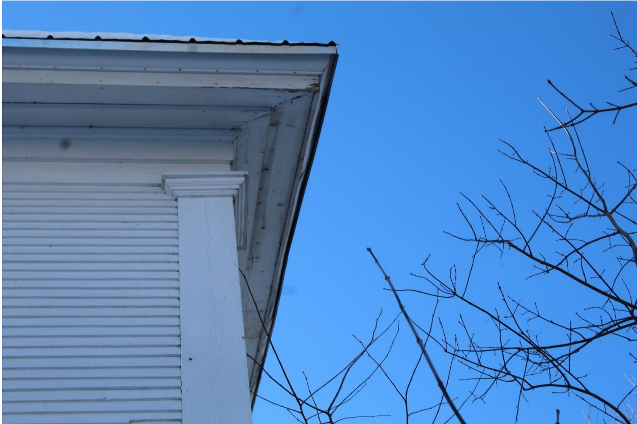
Vermont_LamoilleCounty_GihonValleyGrangeHall_0005: Exterior, northern elevation showing detail of rear pilaster. Camera facing southwest.
