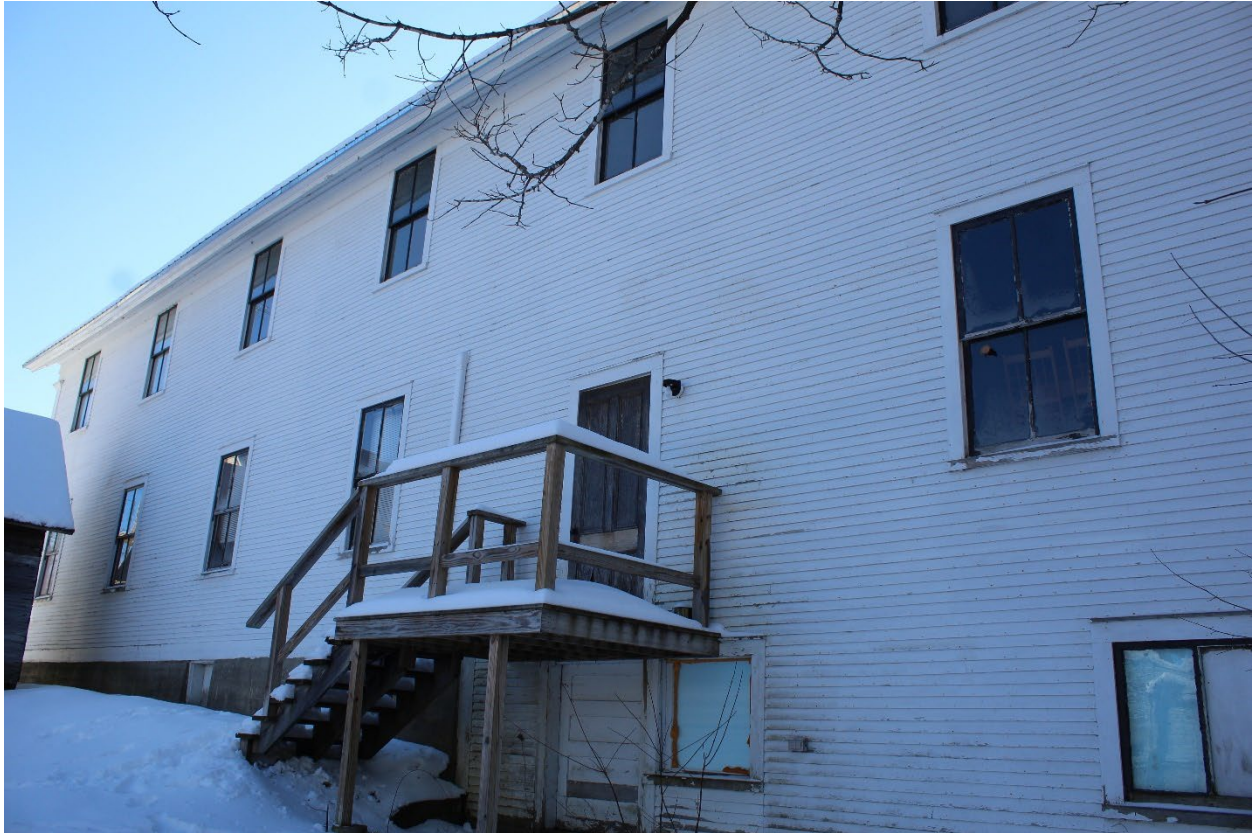
Vermont_LamoilleCounty_GihonValleyGrangeHall_0004: Exterior, northern elevation towards the rear of the building. Camera facing southwest.
