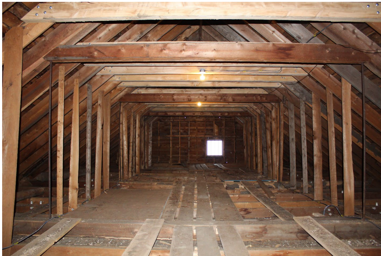
Vermont_LamoilleCounty_GihonValleyGrangeHall_0017: Interior, attic showing the framing of the Gihon Valley Grange Hall's roof. Camera facing northwest.
