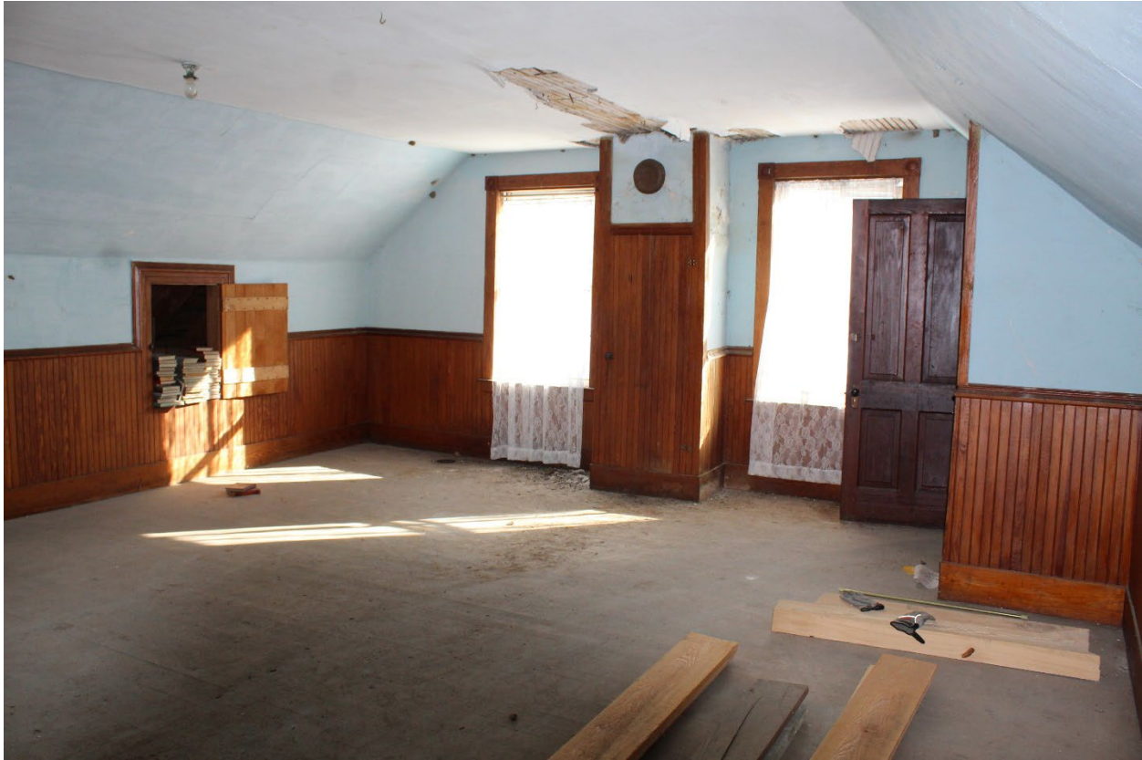
Vermont_LamoilleCounty_GihonValleyGrangeHall_0016: Interior, attic showing the finished room with its original finishes. Camera facing east.
