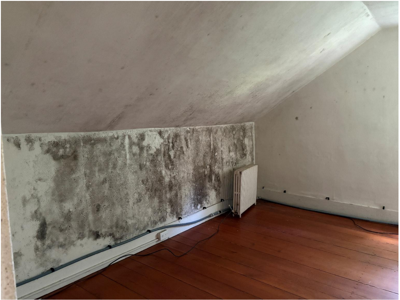
Image 29: Southeast upstairs room; the knee wall shows mold. Looking southeast.
