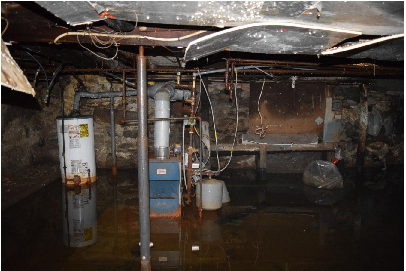
Image 35: View of the basement, flooded with at least 1' of water. Looking to the south wall from the central staircase.
