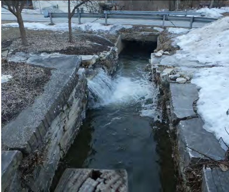
Remnants remain of the marble sluiceway that fed the water to the mills.
