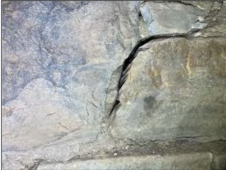
Figure 65. Large void between two interior stones.
