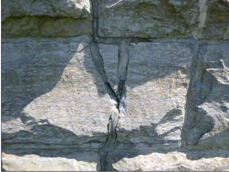
Figure 46. Detached and failed cementitious crack repair (Credit: Vertical Access).
