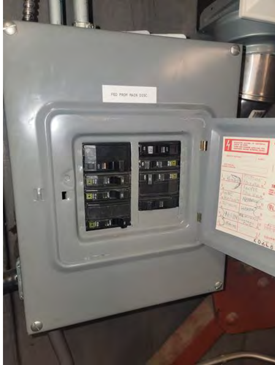
Figure 6. Elevator machine room panel
