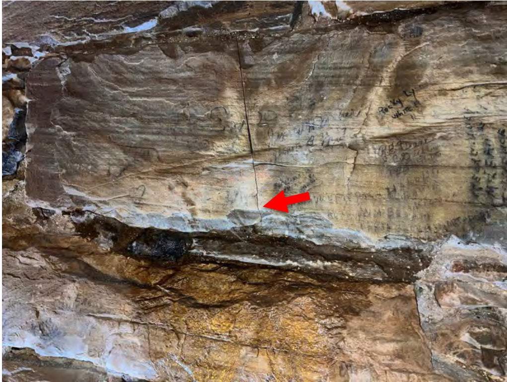
Figure 25. Leak observed as a result of spray testing below crack at interior stone.
