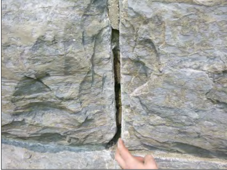
Figure 48. Typical open joint at upper portion of monument. Note mortar at top of joint is deteriorated but remains firmly in place. (Credit: Vertical Access.)
