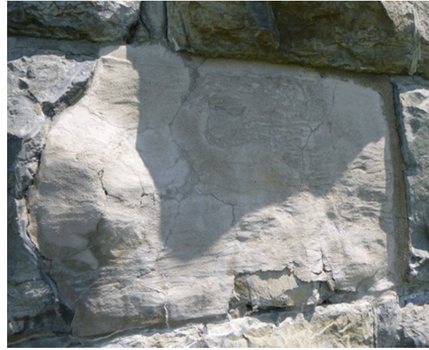
Image 84. Cracked and failed parge coat applied over the face of a stone. Vertical Access
