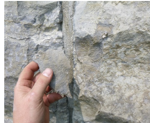
Image 78. Spall removed from the exterior stone masonry. Vertical Access
