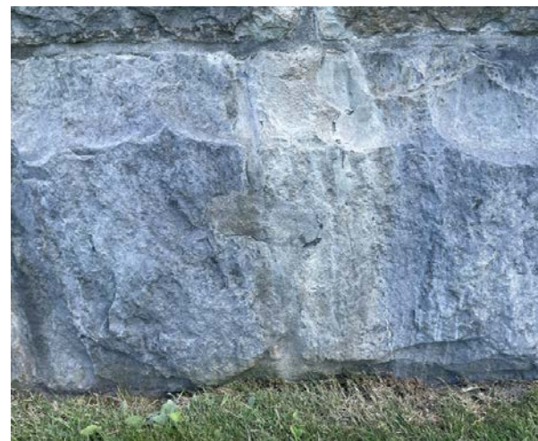
Image 81. Heavy accumulation of carbonate material leached from a cracked and deteriorated mortar joint. Jablonski
