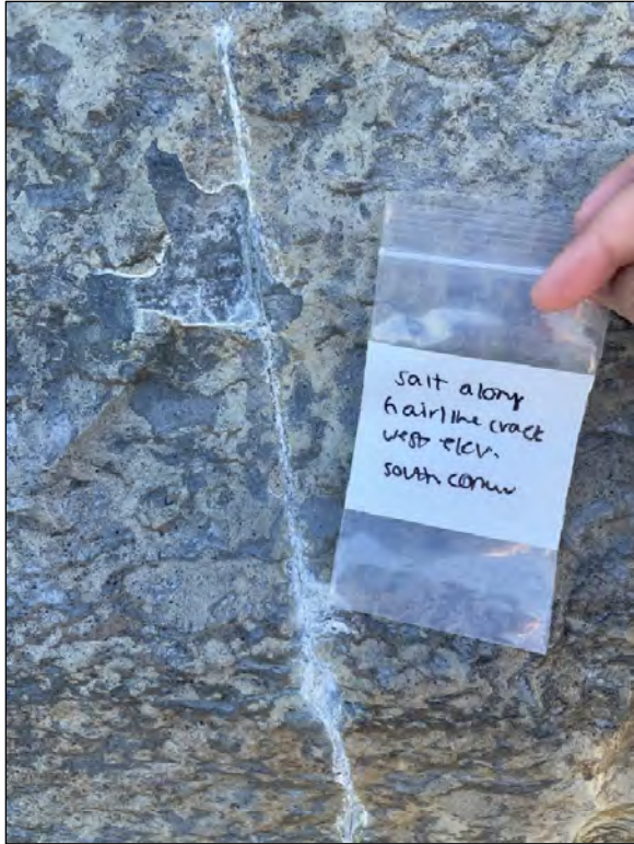
Figure 53. White-colored calcium carbonate deposit along hairline crack.
