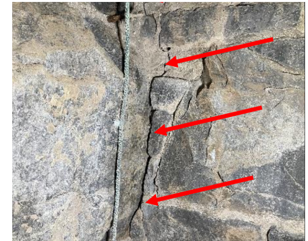
Image 41. Path of separation at the corner. Jablonski
