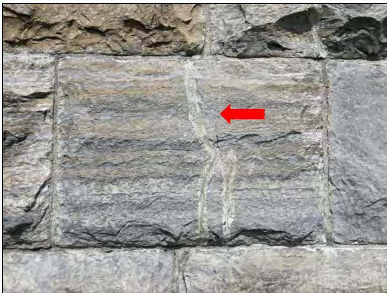
Figure 45. A previously repaired crack with a fresh hairline crack (indicated) extending from the repair.
