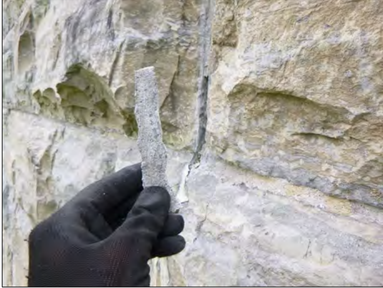
Figure 51. Failed mortar joint at upper portion of monument removed (Credit: Vertical Access).
