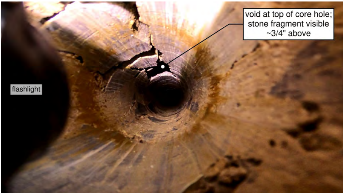
Figure 21. GoPro photo of the masonry between the interior and exterior face wythes (approx. depth of photo = 22" into wall) at CORE-NORTH after the Goodman Jack testing. This portion of the wall was not loaded with the Goodman Jack due to the already present voiding. Figure 22 shows a closer view of the void called out by the annotation in this photo.
