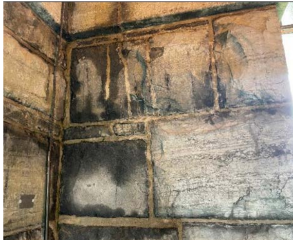
Image 39. Discoloration due to dampness in the corners of the observation platform. Jablonski
