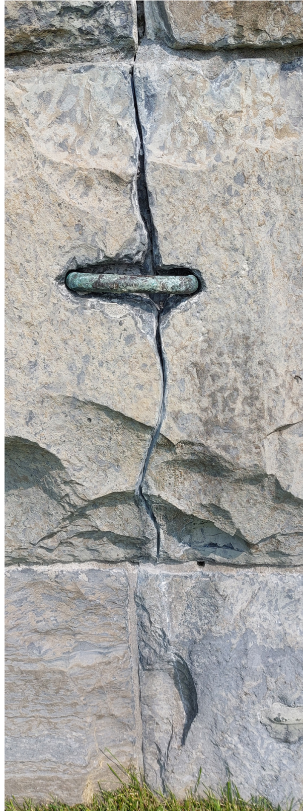
Image 75. Bronze staple condition through crack. Easton Architects
