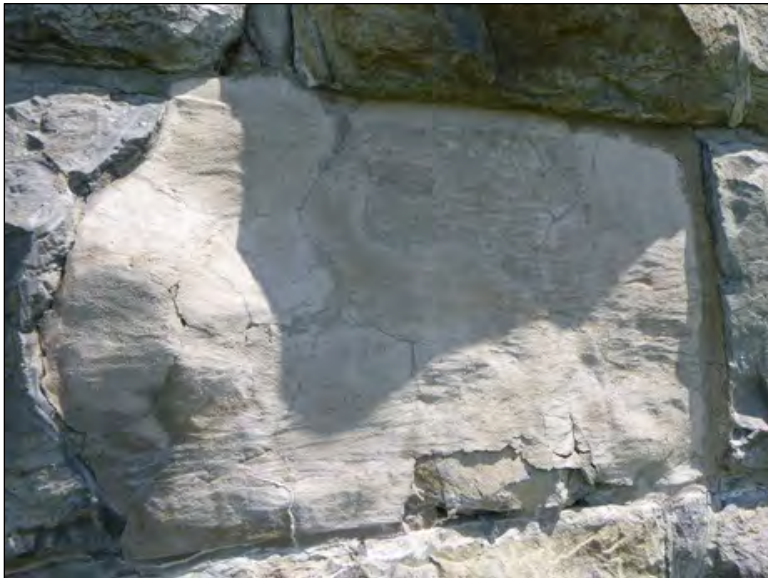
Figure 39. Cracked and failed parge coat applied over the face of a stone (Credit: Vertical Access).
