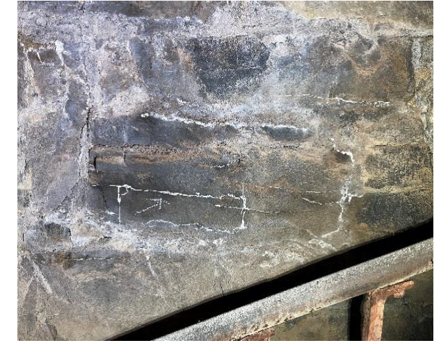
Image 90. Cracks creating an "alligatored" pattern, with white efflorescence along the cracks. Jablonski
