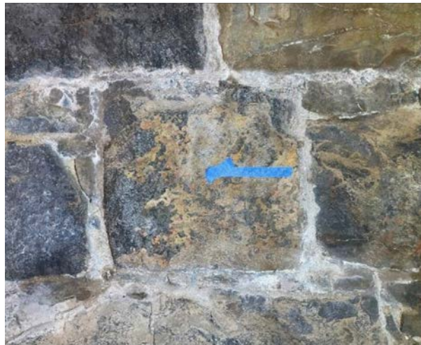
Image 38. Rust-colored crust on the surface of the dark gray stone. Jablonski
