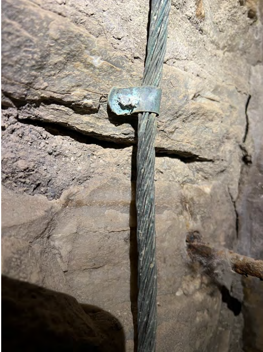
Image 7. As the conductors travel through the monument the condition of the fasteners gets progressively worse. Towards the lower half of the tower many of the fasteners are mostly corroded and are only loosely holding to the inside wall of the tower. This report recommends addressing the moisture issues in the tower then replacing all, or at least the bottom half of the conductor fasteners in the tower.
