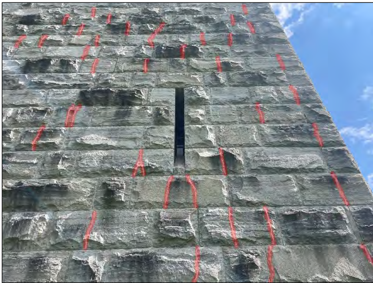
Figure 43. Exterior of monument with cracks highlighted in red. Note that most cracks fall below a vertical mortar joint.
