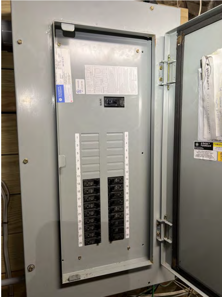
Image 9. There is no surge protection on the main electrical service panel in the monument. Surge protection is required for a complete lightning protection system on all incoming power and communication lines.
