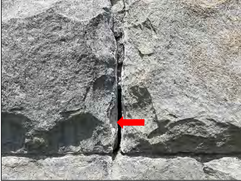
Figure 52. Residue from a previous caulking campaign (indicated) observed below a repointing campaign employing hard, Portland cement-rich mortar that has detached and failed.
