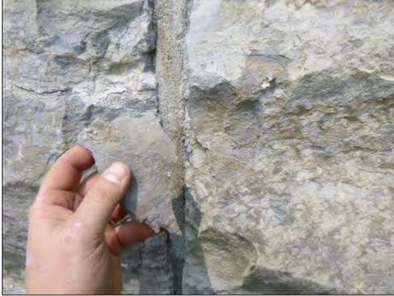
Figure 36. Spall removed from the exterior stone masonry (Credit: Vertical Access).
