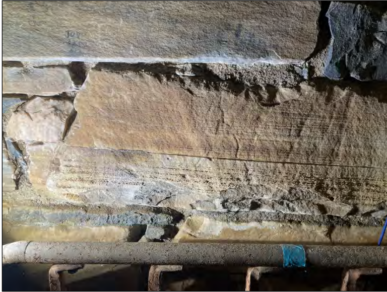
Figure 63. A single, horizontal crack follows the natural foliation of an interior marble unit.
