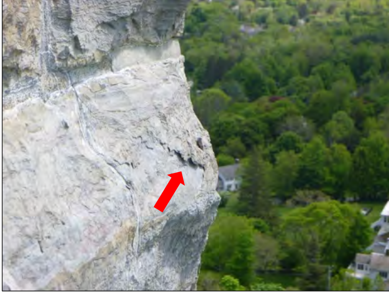
Figure 41. Scaling (indicated) in a stone at the upper portion of the monument (Credit: Vertical Access).
