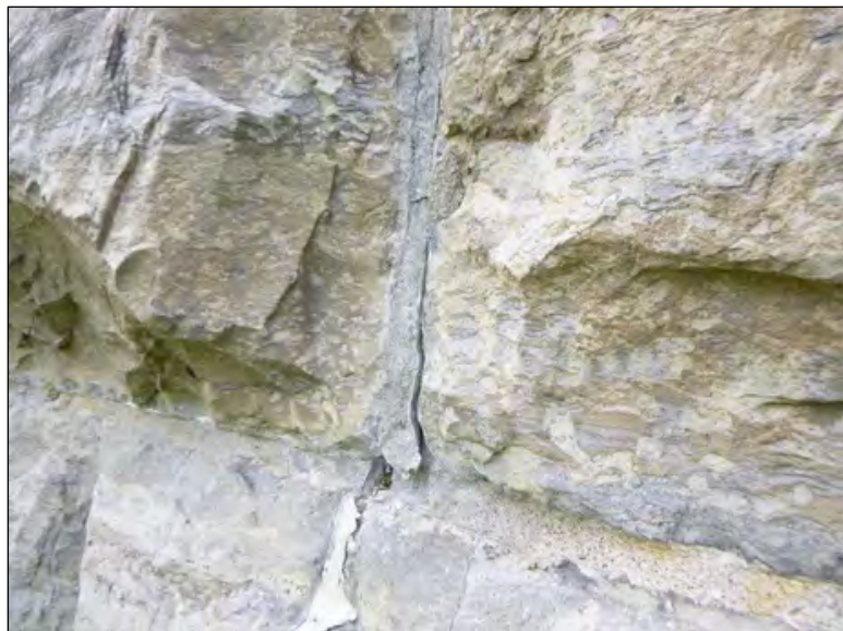
Figure 50. Failed mortar joint at upper portion of monument, possibly resulting from the use of incompatible repointing mortar (Credit: Vertical Access).
