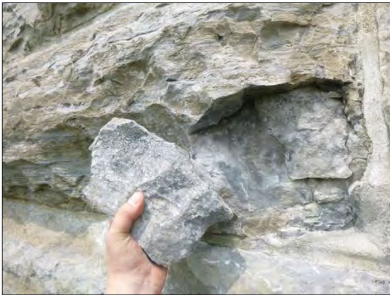
Figure 37. Spall removed from the exterior stone masonry (Credit: Vertical Access).
