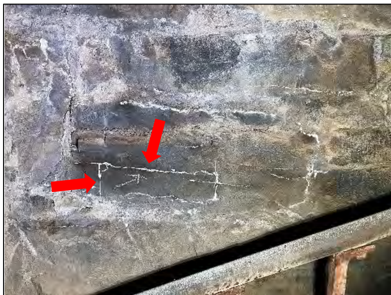
Figure 24. Orthogonal cracks (indicated) in an interior breccia unit. White efflorescence or carbonate deposits occur along the cracks.
