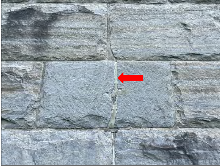
Figure 42. Exterior crack (indicated, repaired with caulk) showing typical vertical orientation and location below mortar joint.
