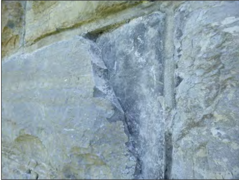
Figure 40. Delamination in a stone at the upper portion of the monument (Credit: Vertical Access).
