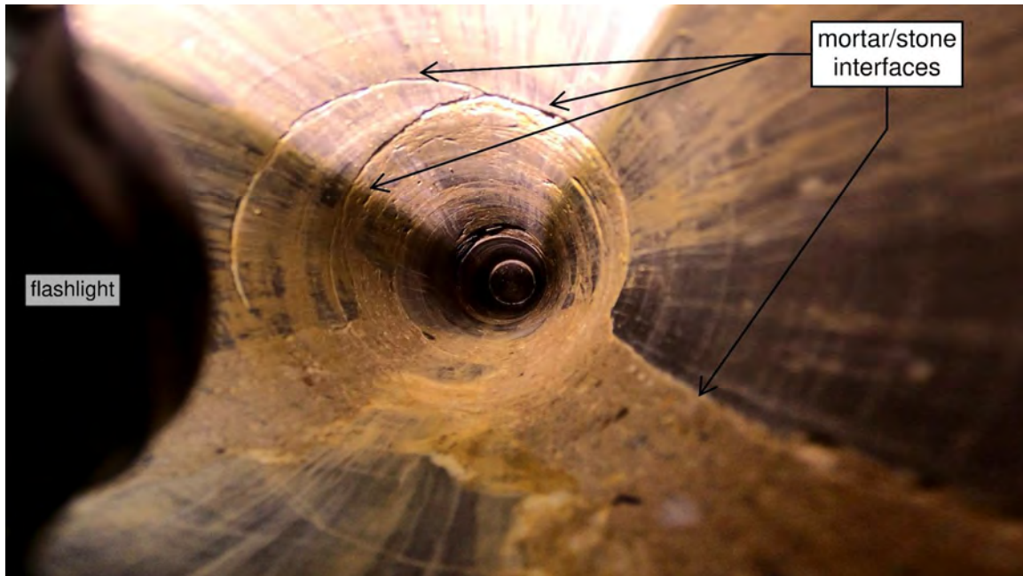
Figure 23. GoPro photo masonry between the interior and exterior face wythes (approx. depth of photo = 40" into wall) at CORE-NORTH after the Goodman Jack testing. Some stone to mortar interfaces appear solid and others show slight separations between stone and mortar.
