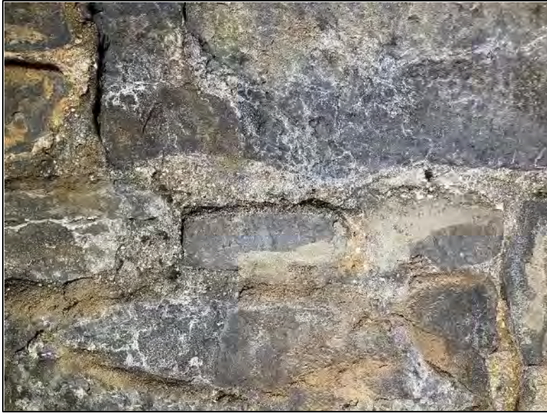
Figure 70. White colored efflorescence on the surface of the stone and mortar joints. Note light brown dust (mortar debris disaggregated by crystallizing salts) accumulating on projections from the stone.
