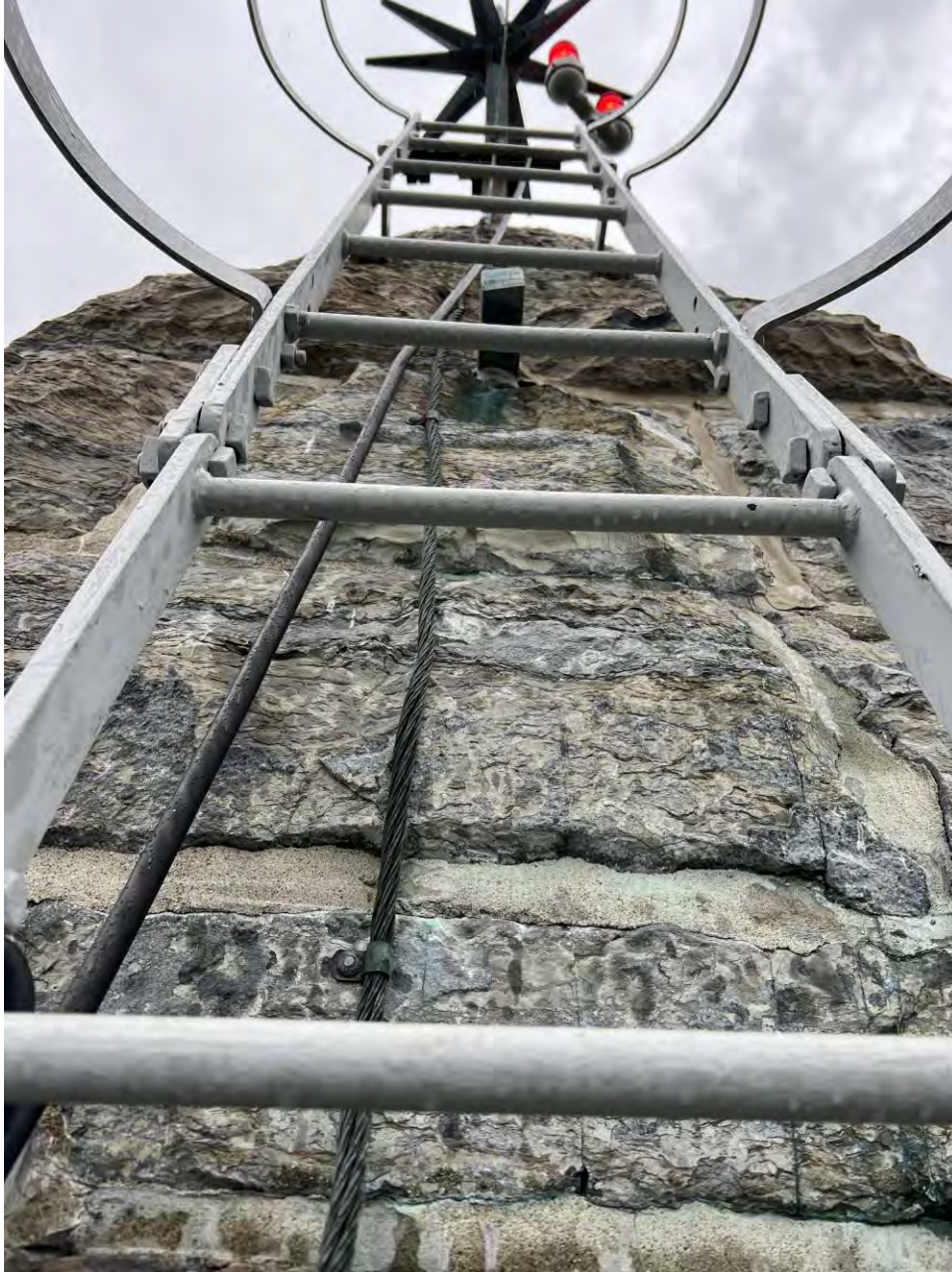
Image 3. The access ladder is directly over the main lightning conductor and is bonded to the lightning protection system at the base of the ladder through a thru bolt into the tower. This report recommends bonding the ladder at the top as well as at the bottom. Also, the platform below the ladder is not bonded into the lightning protection system. This report recommends that the platform be bonded into the system as well.
