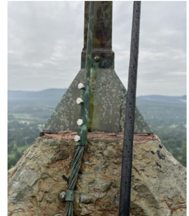
Image 60. Bolted connection from air terminal to class II copper lightning conductor. Smokestack Lightning.
