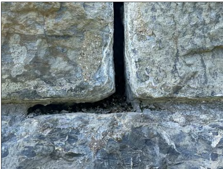
Figure 47. Detail of a typical open joint showing accumulation of crumbly mortar and debris at bottom of joint.
