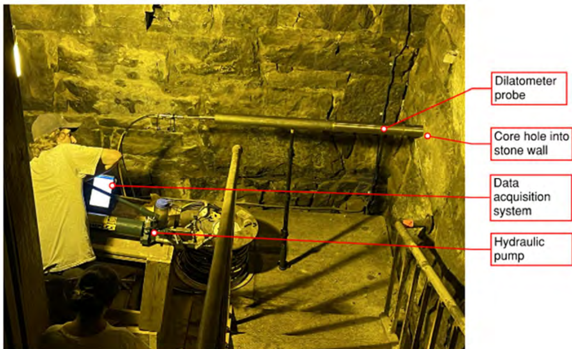
Figure 41. Configuration of goodman jack testing at interior landing 26 on the north wall.
