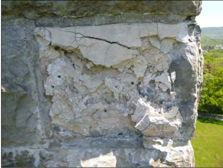
Figure 38. Cracked and spalled cementitious patch repair (Credit: Vertical Access).
