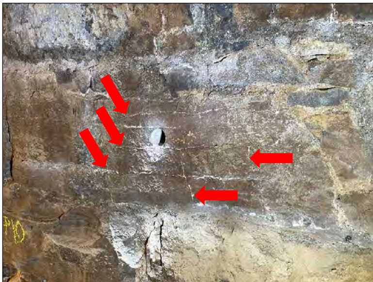
Figure 62. Orthogonal cracks (indicated) in an interior breccia unit.
