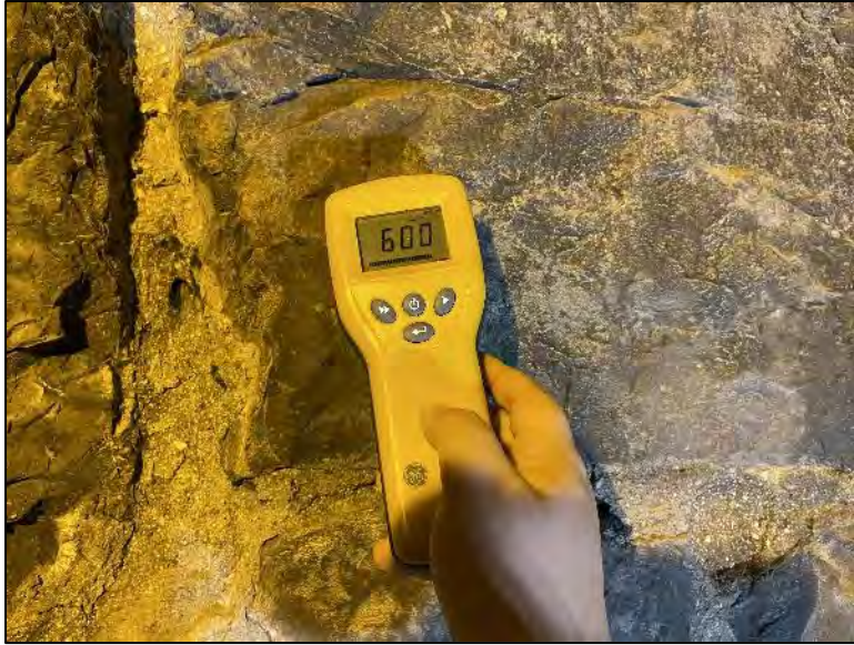
Figure 57. A high, 600 moisture reading taken at the interior stone.
