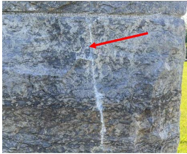
Image 51. Shallow spall. Jablonski
