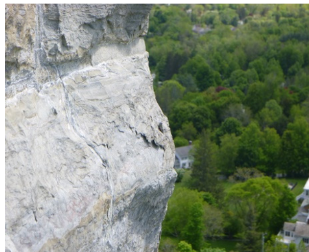
Image 80. Scaling in a stone at the upper portion of the monument. Vertical Access
