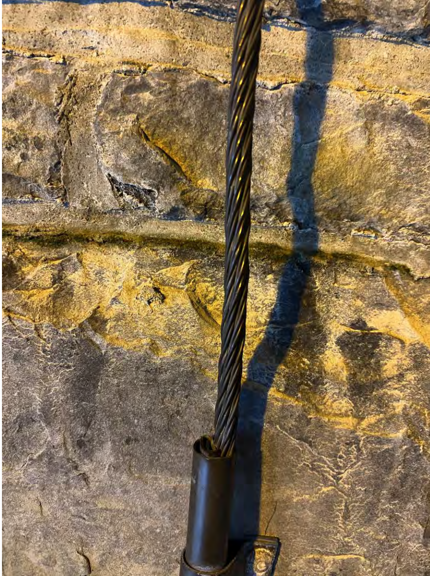
Image 6. At the publicly accessible levels of the monument the conductors are protected by a copper conduit. To keep continuity between the conduit and the conductor a copper wedge is placed into the top of the conduit. This wedge is visible on some of the conduits but not the others. This report recommends confirming or bonding each copper conduit to the lightning protection conductor at the top and bottom of the conductor as required by the lightning protection standards.
