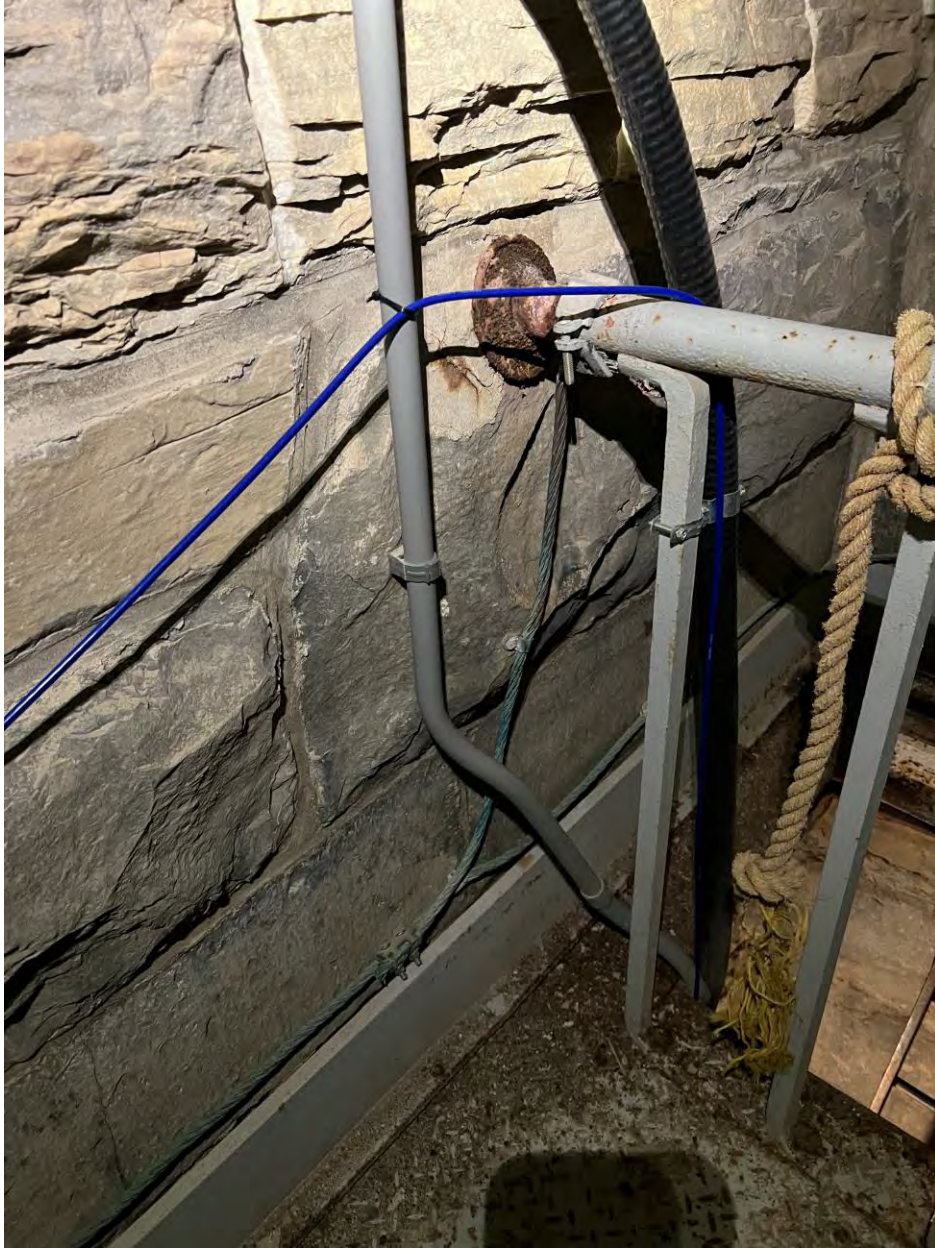
Image 5. The patinaed copper wire runs horizontally and connects the 2 opposite conductors at 4 levels. This intermediate connection is required per NFPA, UL and LPI standards for structures of this height. The bond to the railing is showing some signs of corrosion.
