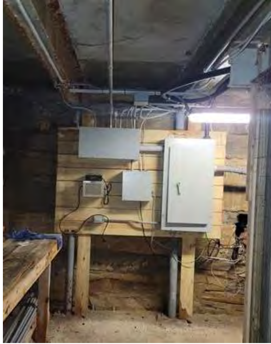
Figure 5. Main Electrical Panel in monument basement
