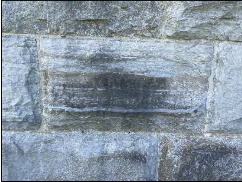
Figure 56. Biological soiling (dark colored material) on surface of an exterior stone.
