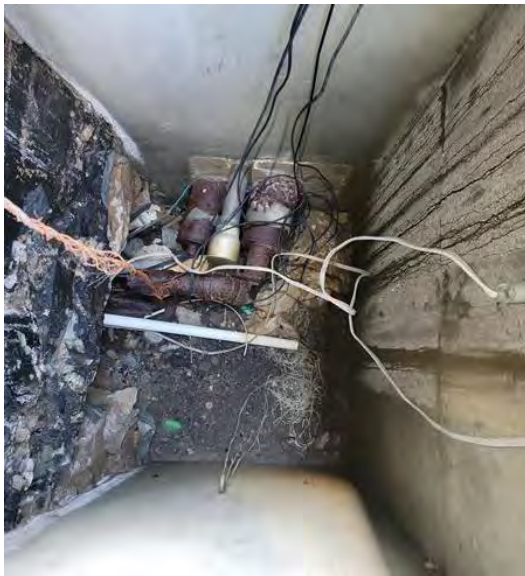
Figure 3. Abandoned piping in pit adjacent to monument
