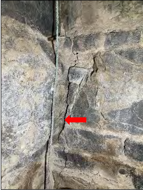
Figure 59. Typical crack (indicated) at interior corner.
