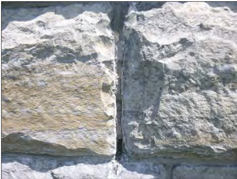
Figure 49. Typical open joint at upper portion of monument. Note mortar at top of joint is deteriorated but remains firmly in place. (Credit: Vertical Access.)
