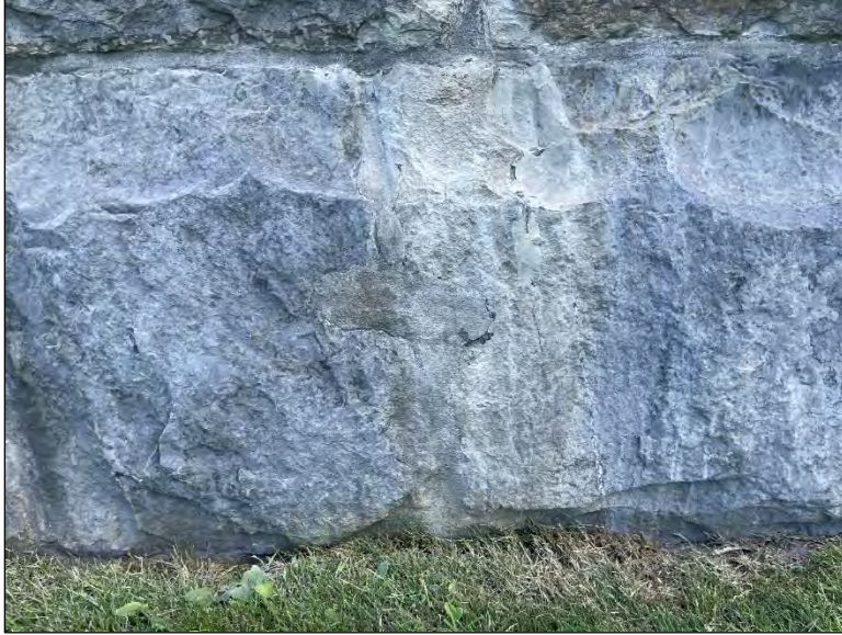
Figure 55. Heavy accumulation of carbonate material leached from a cracked and deteriorated mortar joint.
