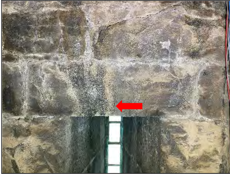
Figure 61. A hairline crack (indicated) through a window lintel resulting from the load of the masonry carried above.
