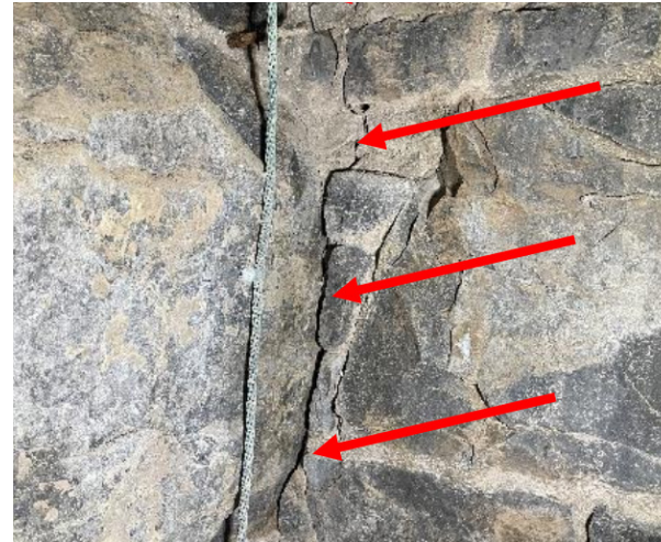
Image 47. Path of separation at the corner. Jablonski
