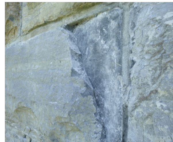
Image 76. Delamination in a stone at the upper portion of the monument. Vertical Access
