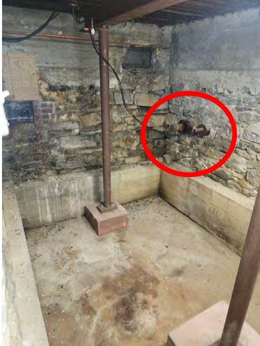
Figure 2. Former boiler room in visitor's center. Note piping cut and capped
