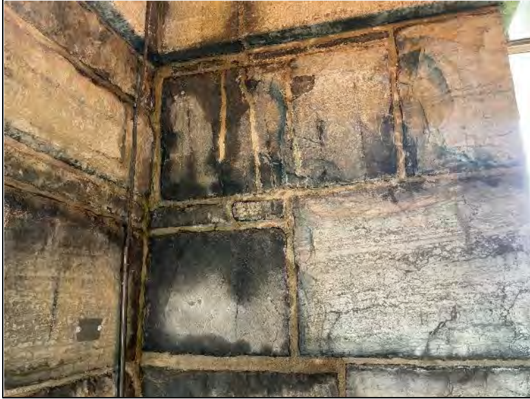
Figure 58. Discoloration due to dampness in the corners of the observation platform.
