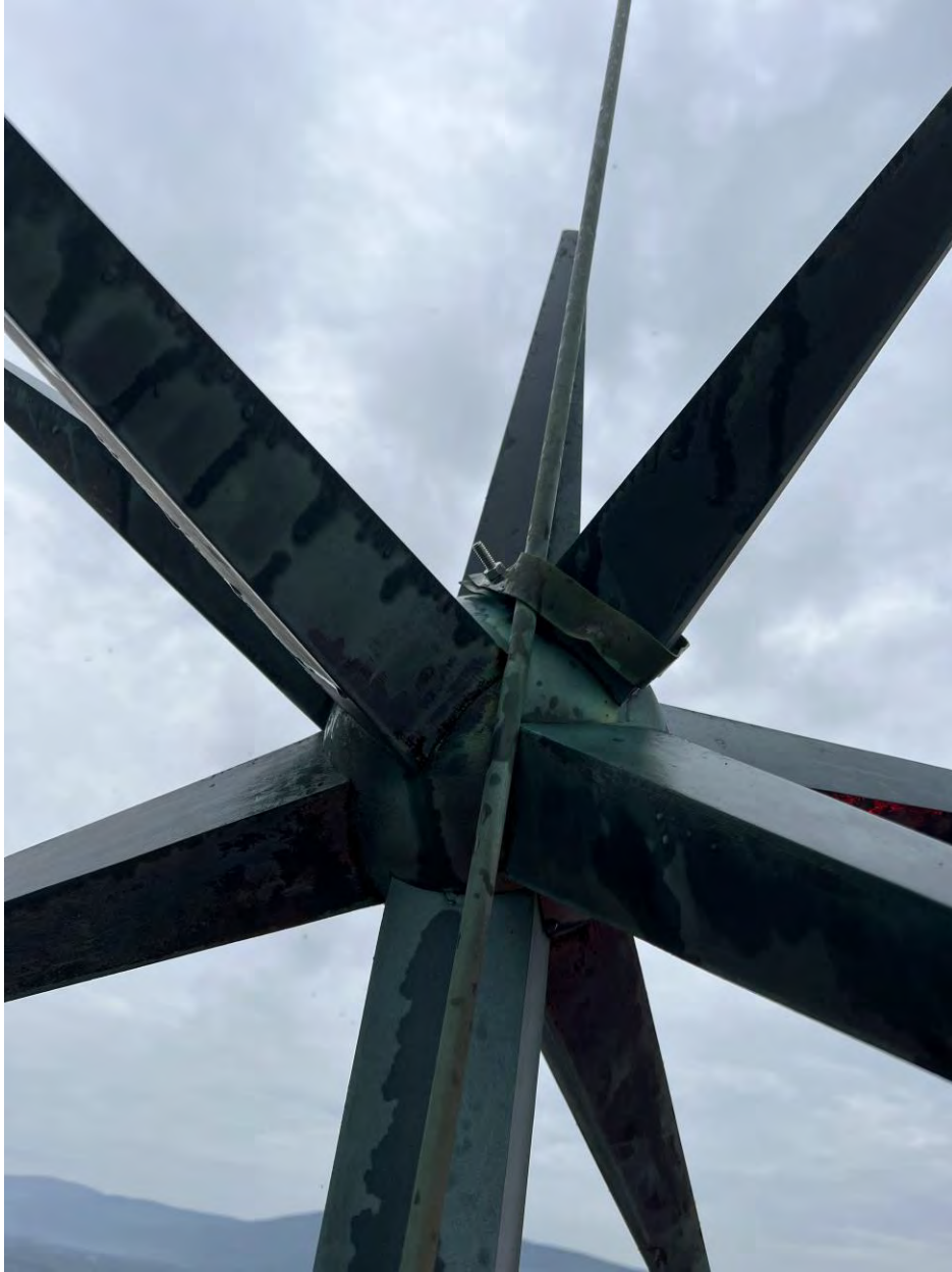
Image 1. ½” diameter class II copper air terminal mounted with bolted copper strapping to star finial. This report recommends a full-size bond between the finial and the air terminal. The strapping currently provides this bond but it is difficult to determine if there is adequate surface area for the connection.
