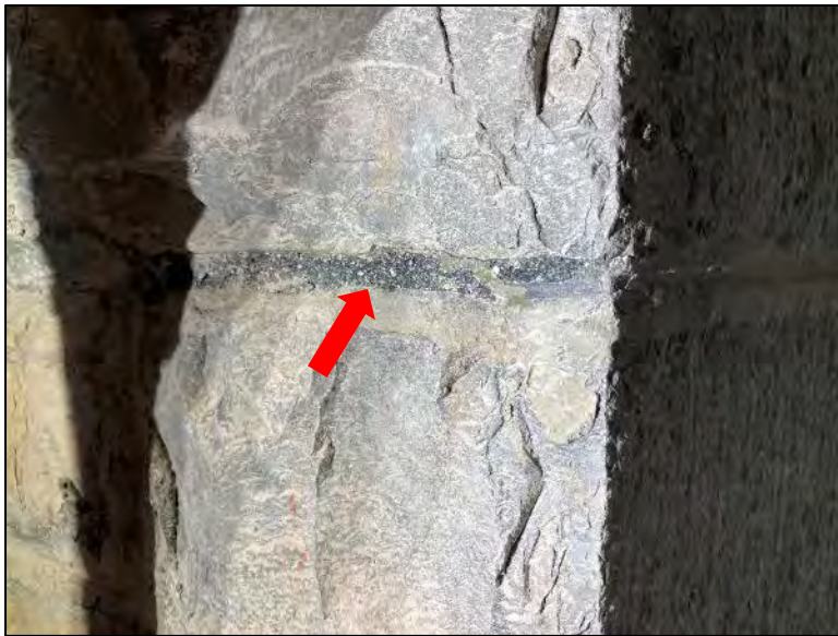
Figure 28. Black-colored pointing mortar (indicated) at interior window return is likely original pointing mortar.
