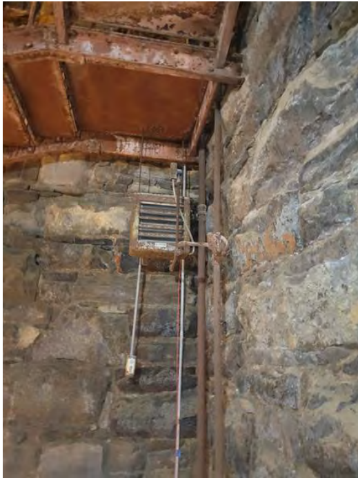
Figure 1. Remnants of abandoned heating system in monument
