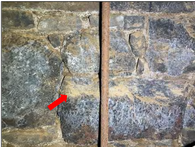
Figure 66. Light brown disaggregated mortar (indicated) coats projecting surfaces of interior stones.
