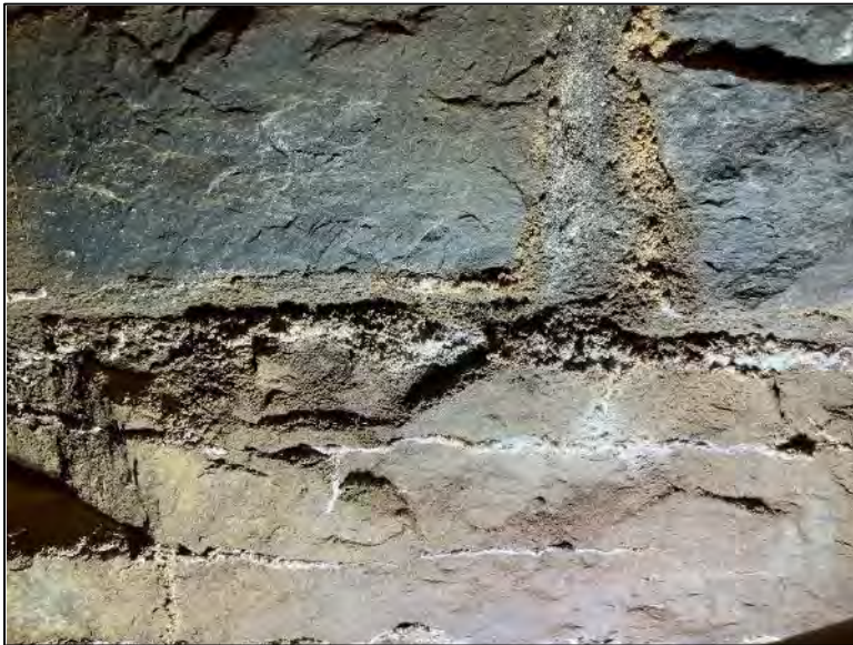
Figure 69. Efflorescence and/or carbonate crusts along cracks and mortar joints.
