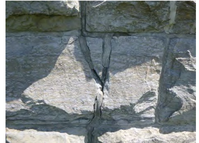
Failing Cement Caulk
