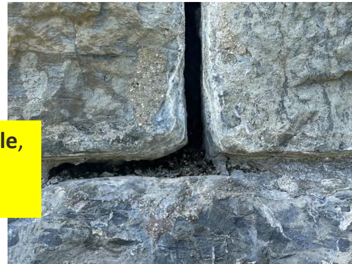
Open joint with crumbly mortar & debris
