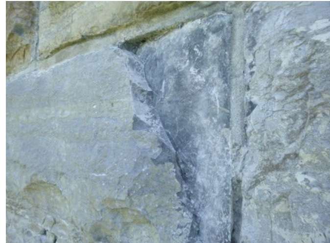
Delamination of stone
