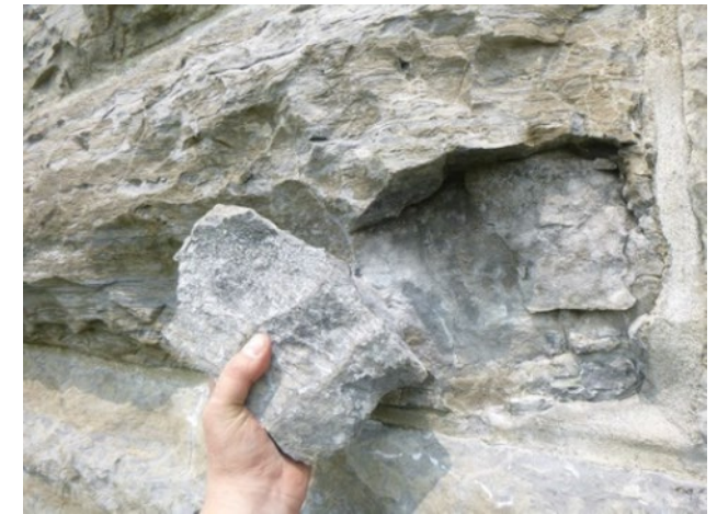
Spalling of Stone
