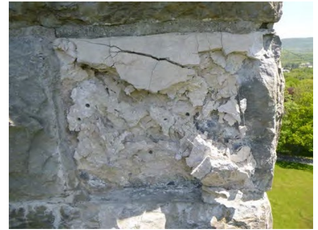
Failing Cement Patch
