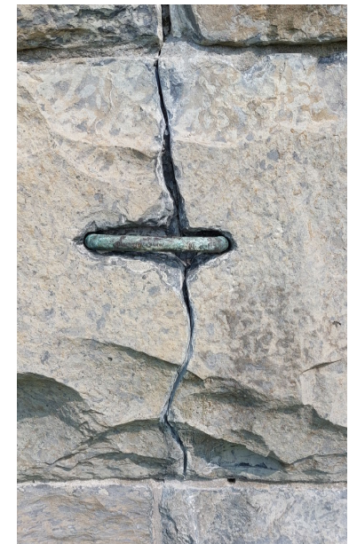
Damage from Metal Anchor Repair
