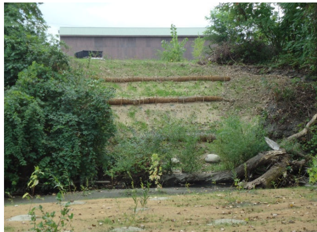
Mass failure after restoration
