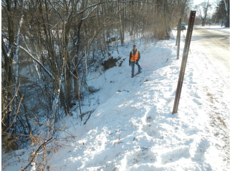
Figure 9: Top of bank failure along Wheeler Road
