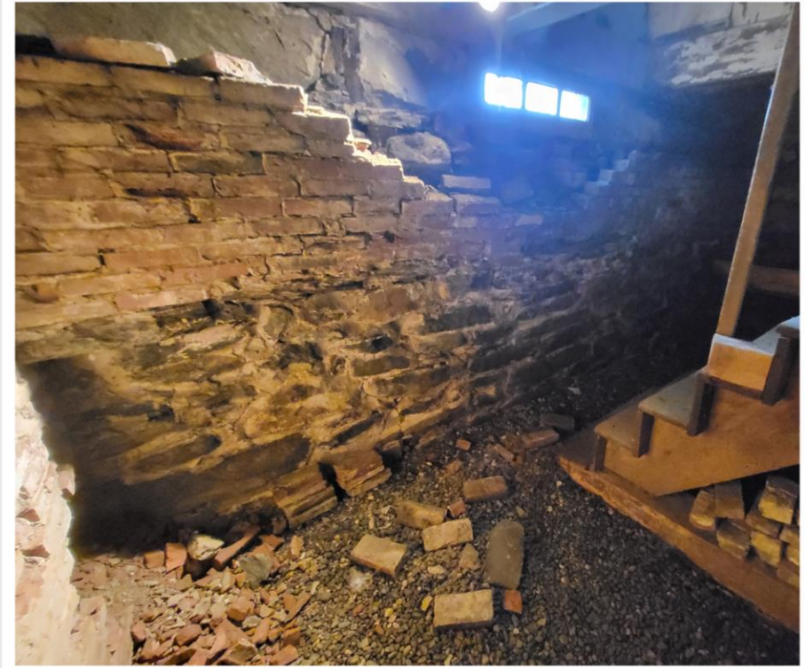
Damp & deteriorated masonry foundation
