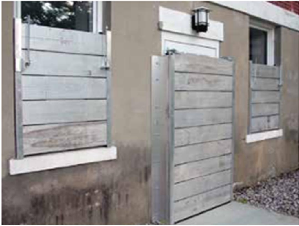
Dry: Water Barrier Temporary barriers with permanent stanchions installed to prevent water from entering
