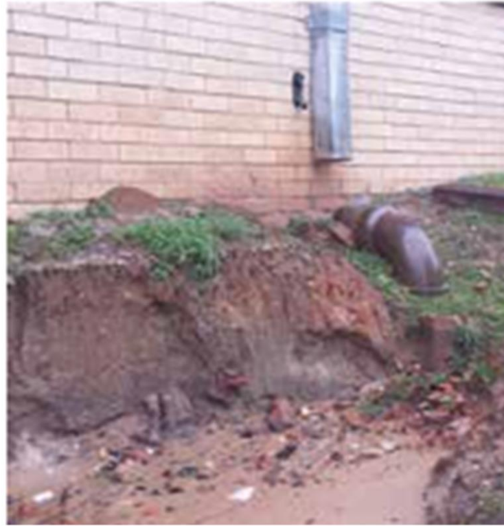
Disconnected downspout & undermined foundation
