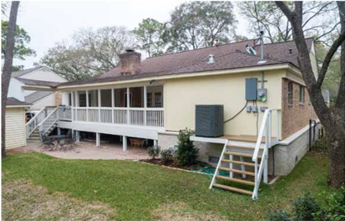
Elevated mechanicals on rear of building
