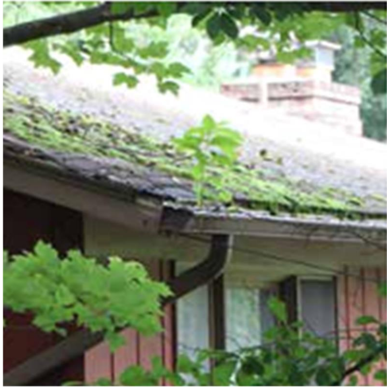
Wet roof and clogged gutters
